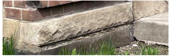
Figure 94. East elevation stone soiling (ERA, 2022).
