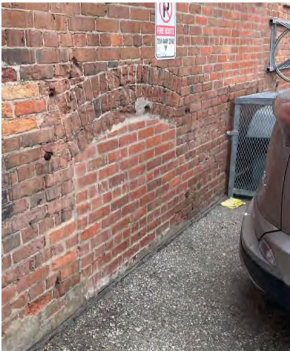
Figure 107. Basement window infill at west elevation with surrounding spalling, parging and holed bricks (ERA, 2022).
