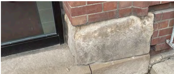
Figure 95. East elevation south entryway base stone soiling and erosion (ERA, 2022).
