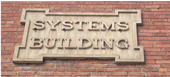
Figure 97. East elevation stone sign soiling (ERA, 2022).
