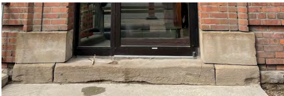
Figure 93. East elevation north entryway base stone and sill with soiling and erosion (ERA, 2022).
