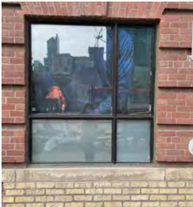
Figure 99. Typical condition of windows at exterior (ERA, 2022).
