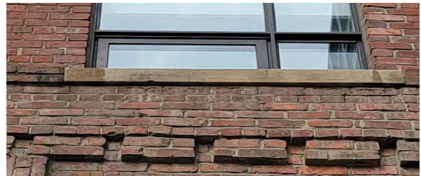
Figure 96. East elevation displaying mortar loss and soiling (ERA, 2022).
