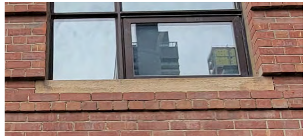
Figure 98. East elevation typical soiling of stone sills (ERA, 2022).
