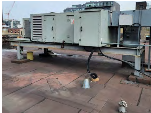
Figure 110. HVAC components on steel structure (ERA, 2022).
