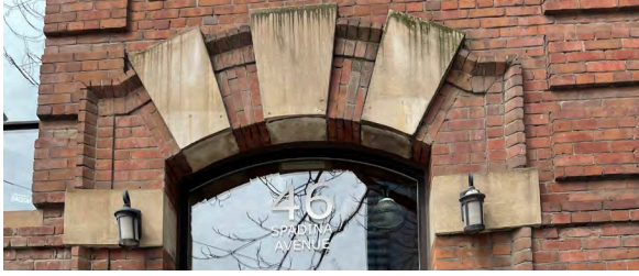
Figure 91. East elevation north entryway key-stones and jambs displaying soiling (ERA, 2022).
