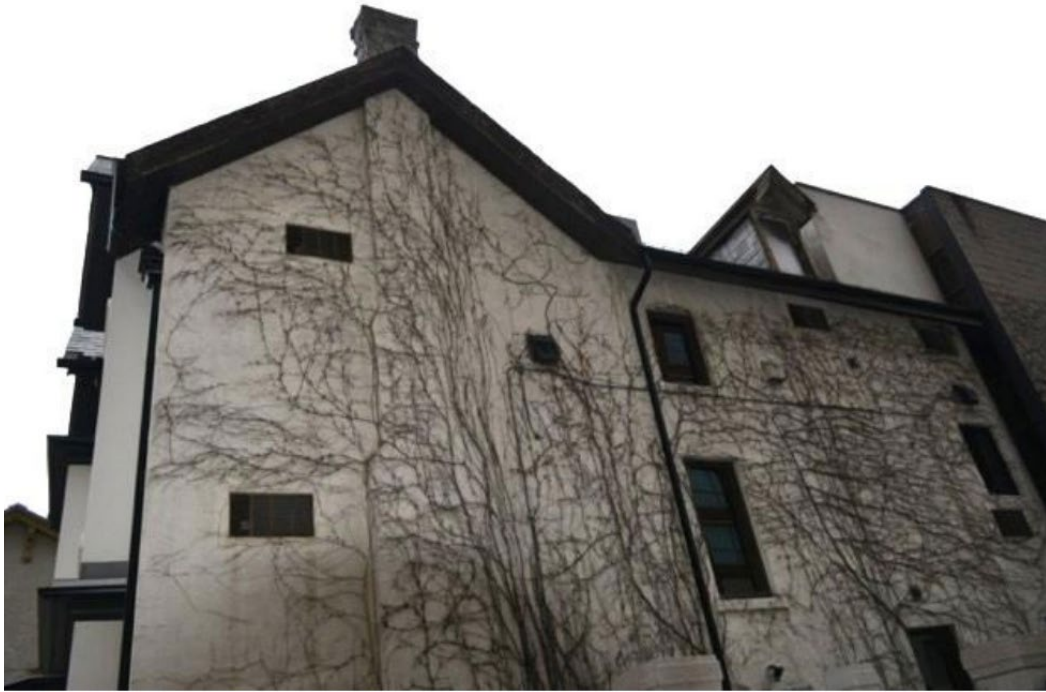
East elevation of 8 Prince Arthur Avenue showing existing windows, chimney, dormer. The proposed dormer is proposed to be removed while the chimney and windows are proposed to be retained and repaired where required (Source: GBCA Architects, 2026)
