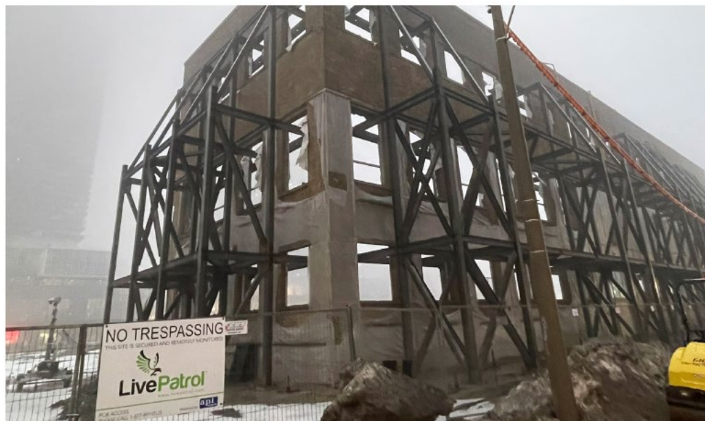
Figure 11: North and west elevation of the Warehouse Building, looking southeast (Giaino + Associates Architects Inc., 2026).
