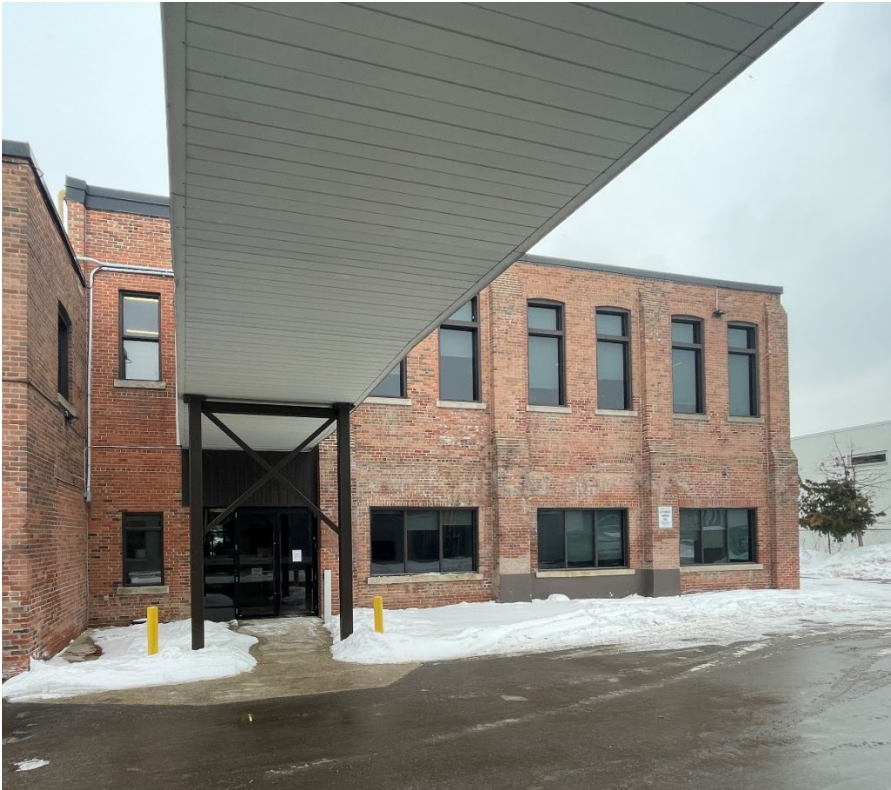
Figure 24. View of the south elevation of the Storage and Anhydrous Ammonia Building, which features wide rectangular window opening at the first storey and paired segmental arch window openings with brick voussoirs at the second storey (Heritage Planning, 2026).
