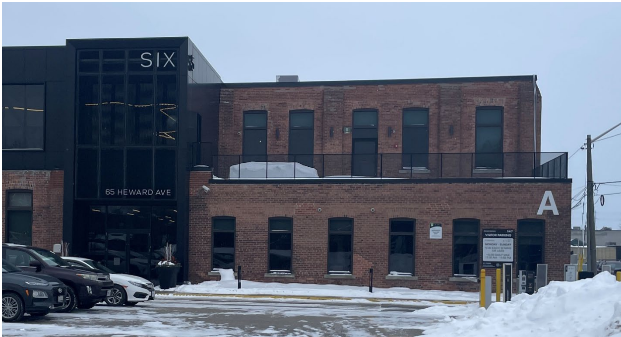
Figure 19. View of the north elevation of the Office and Aqua Ammonia Building, showing the second storey above the north wing, which features 3 bays that are divided by brick pilasters and feature segmental arch window openings with brick voussoirs (Heritage Planning, 2026).
