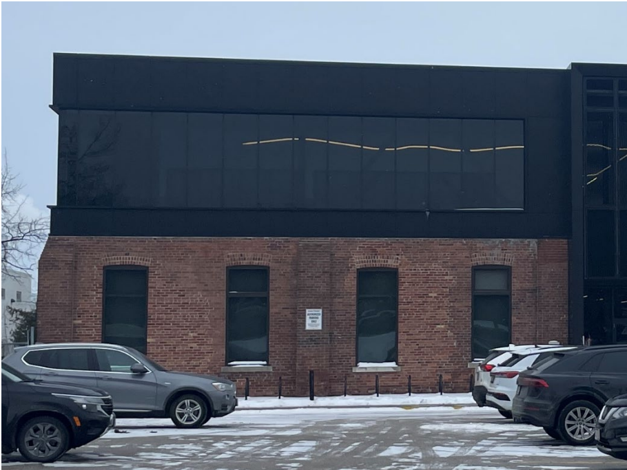
Figure 25. View of north elevation of the Storage and Anhydrous Ammonia Building, which features paired segmental arch window openings with brick voussoirs at the first storey (Heritage Planning, 2026).
