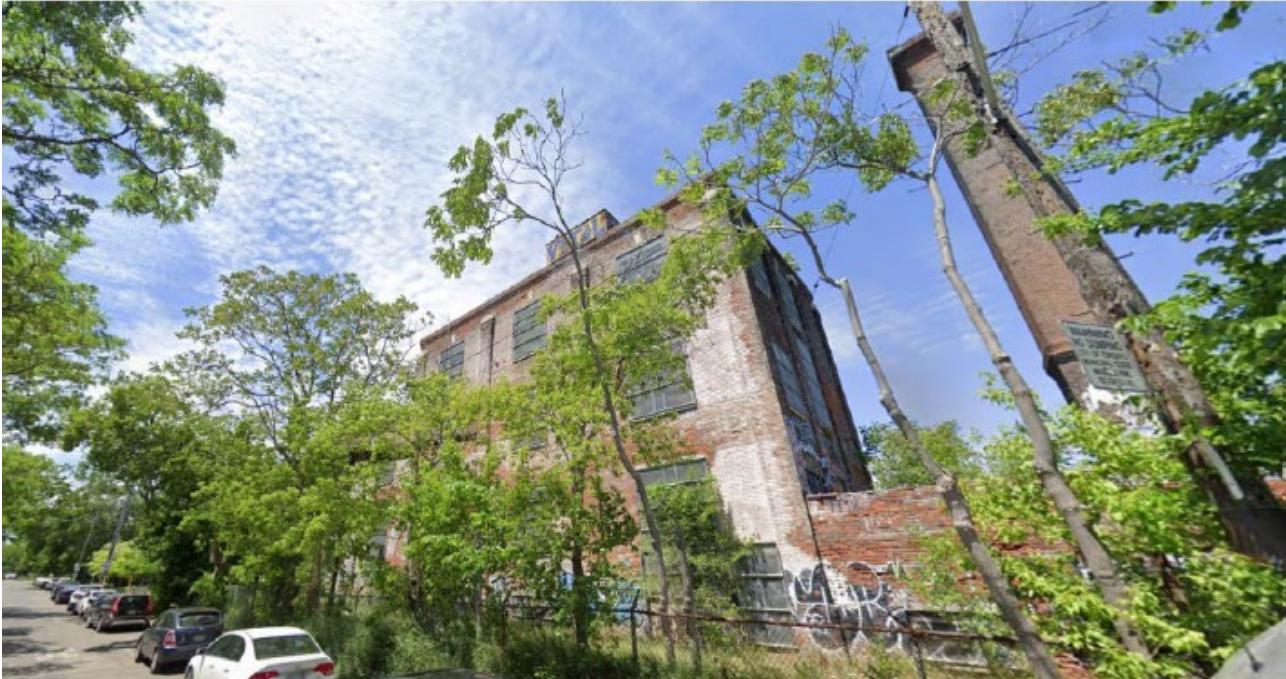
View of the southeast elevation, showing Building B at 40 Wabash Avenue and Building C with its chimney stack (SBA, 2024).
