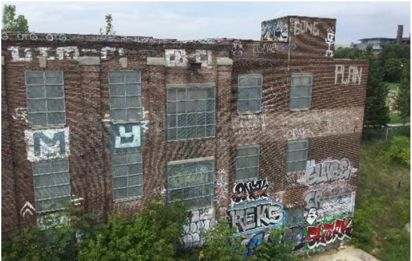
View of the east elevation, showing Building D on the left and Building E (not designated) directly north of the brick pilasters at 40 Wabash Avenue (SBA, 2024).
