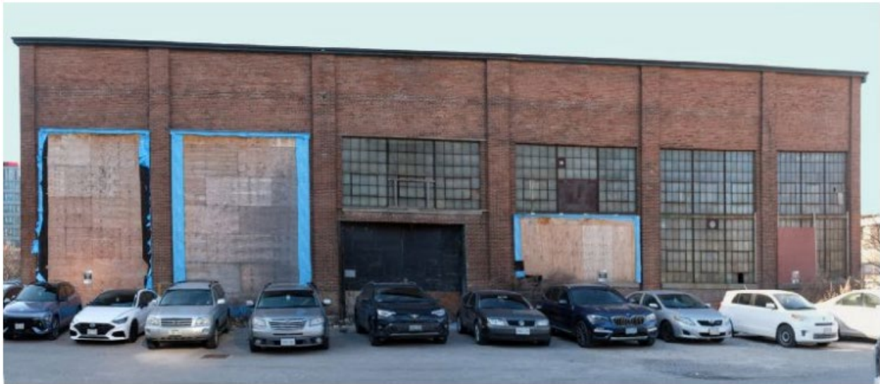
Figure 5: East elevation of 153 Eastern Avenue (Cleaning Room building), looking west (Philip Goldsmith Architect, 2025).
