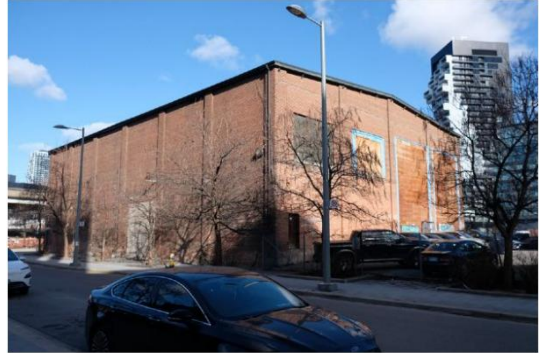
South and west elevation of 153 Eastern Avenue (Cleaning Room building), looking northeast (Philip Goldsmith Architect, 2025).
