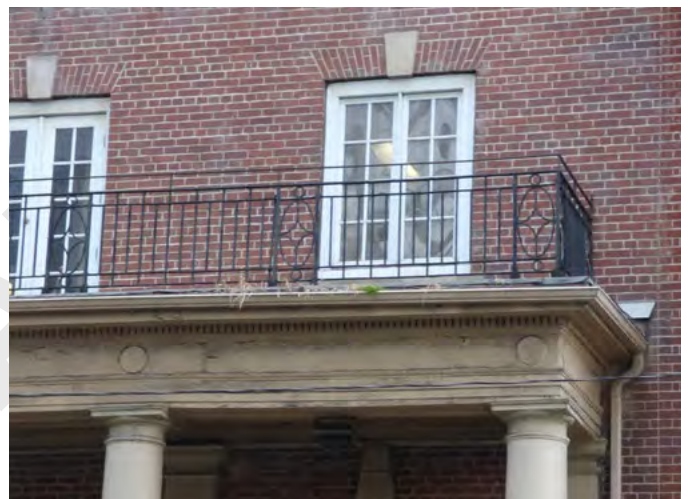
30. Vegetation at gutter and condition of (non-original) balcony railing at roof of portico (ERA, December 2025)
