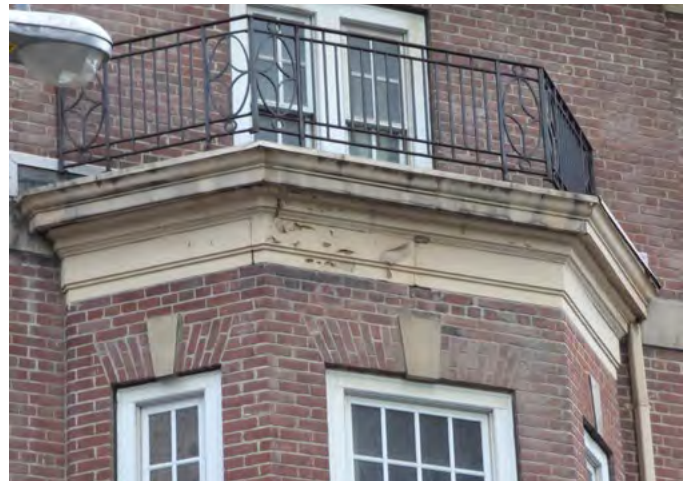
29. Condition of railing at roof of projecting bay (ERA, December 2025)
