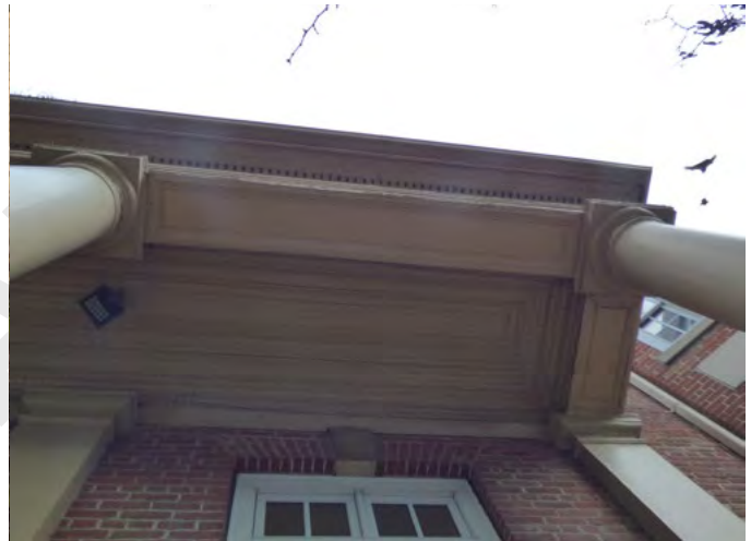
19. Condition at underside of beams and soffit, entrance portico. (ERA, December 2025)
