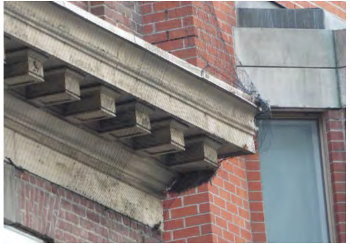
32. Condition of galvanized iron cornice and added bird netting (ERA, December 2025)
