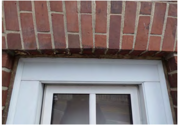
25. Poor condition at sealant at basement window (ERA, December 2025)
