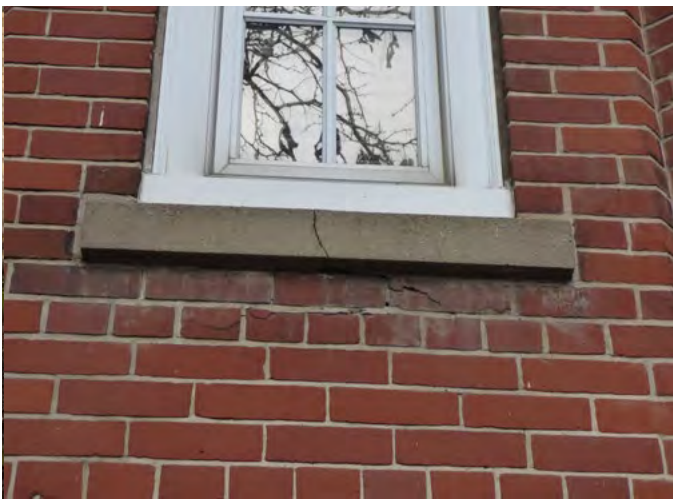
9. Cracked artificial stone sill and cracked brickwork below (ERA, December 2025)
