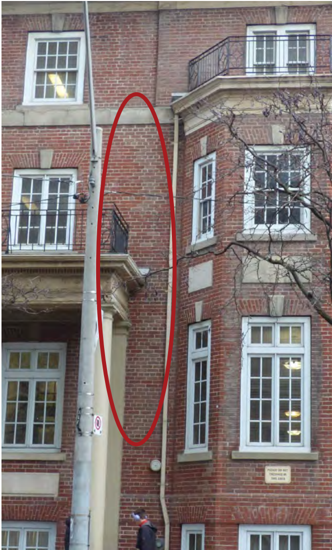
8. Example of previous selective replacement brick surrounding the east portico (ERA, December 2025)
