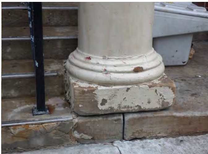
21. Poor condition at replacement concrete steps (ERA, December 2025)
