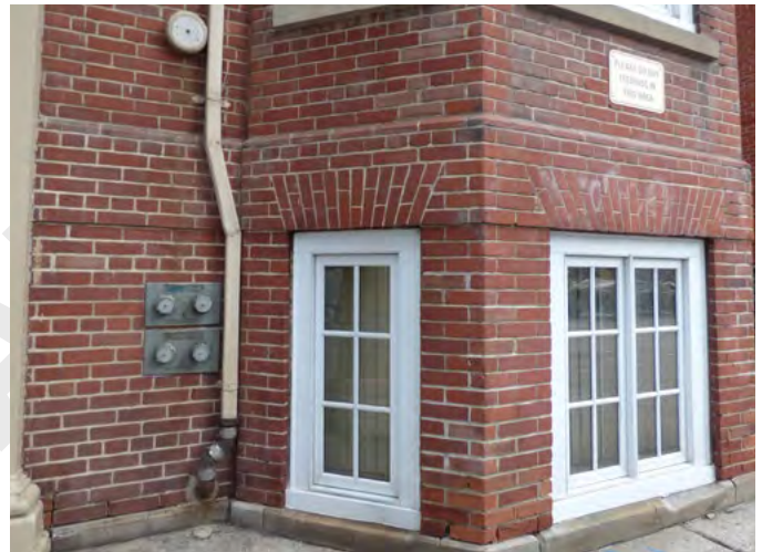
3. Open joints at base, and selective areas of repointing and replacement bricks. (ERA, December 2025)
