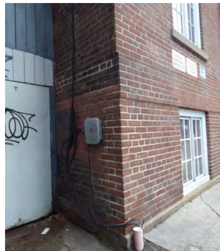
43. Previous rebuilding at base of southwest corner, termination of brick plinth (ERA, December 2025)
