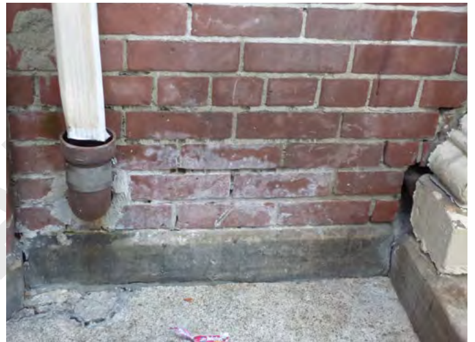
7. Open joints and efflorescence at base of downspout, hole/missing brickwork behind base of wood pilaster (ERA, December 2025)
