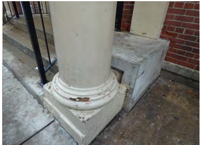
20. Example of rotted wood at missing paint, base of wood column, and condition of later concrete stairs (ERA, December 2025)
