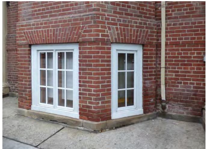
4. Open joints and chipped stone at base plinth, open joints at first courses of brick, and selective areas of repointing and replacement bricks (ERA, December 2025)
