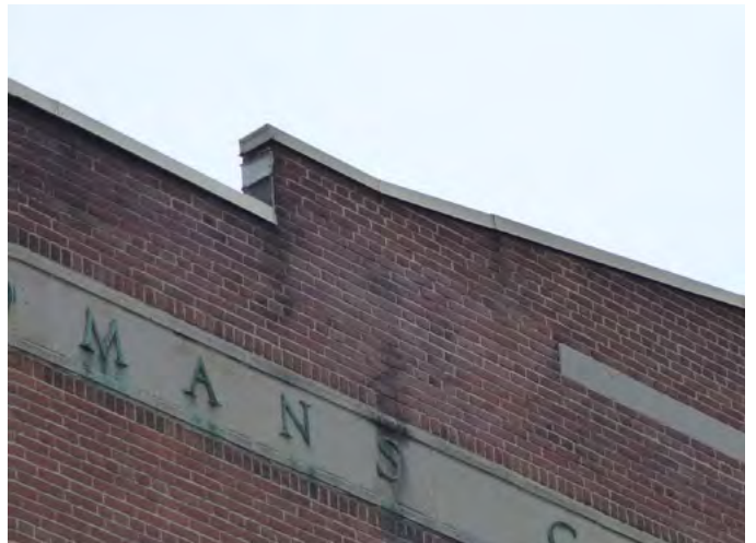
34. Condition of later parapet flashing and bronze letters (ERA, December 2025)
