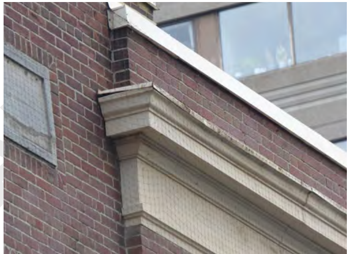
33. Condition of galvanized steel cornice at top of flat bay (ERA, December 2025)
