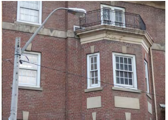
17. Soiling and chipped paint at artificial stone banding and cornice, and typical condition of artificial stone accents (ERA, December 2025)
