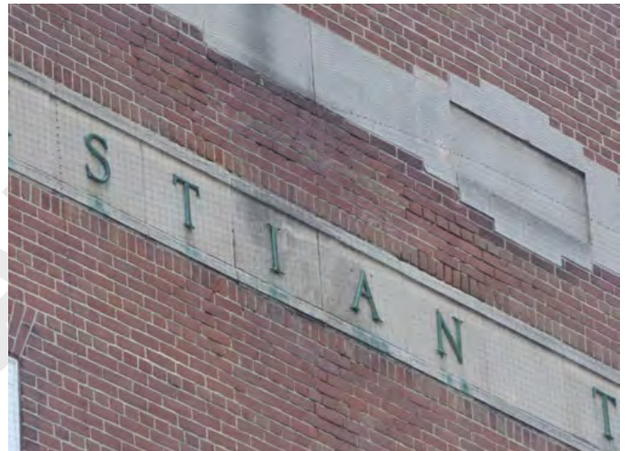
14. Condition of decorative artificial stone units at parapet, including metallic staining from bronze letters (ERA, December 2025)
