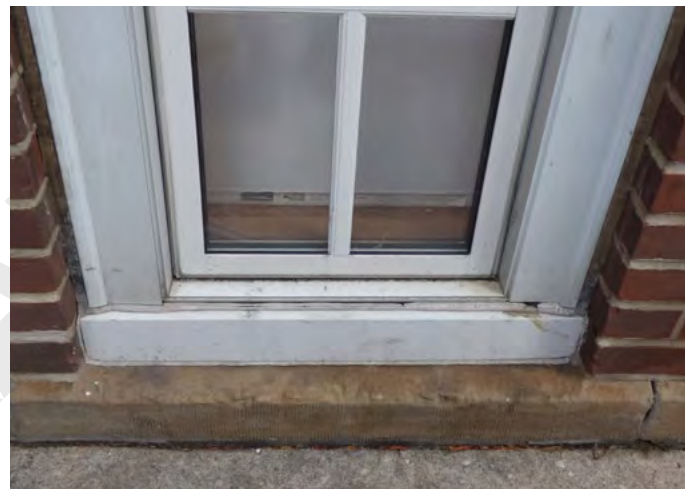
27. Poor condition at sealant at basement window (ERA, December 2025)
