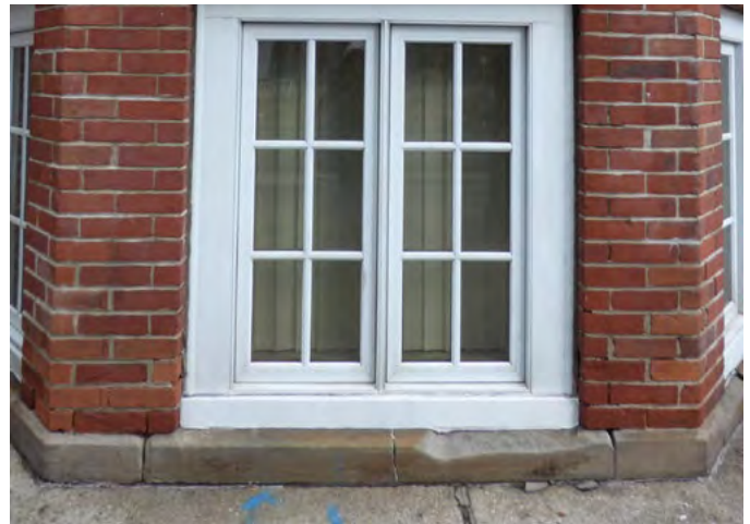
10. Open joints and chipped edge at stone plinth (ERA, December 2025)
