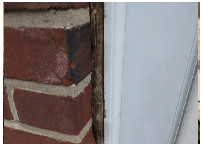
28. Poor condition at sealant at basement window (ERA, December 2025)
