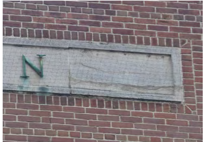
13. Previous patch at artificial stone panel (ERA, December 2025)
