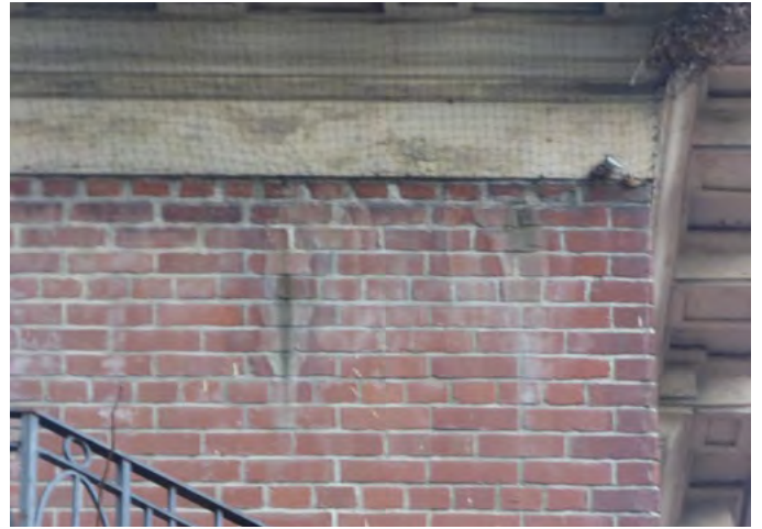
6. Example of soiled brick below cornice (ERA, December 2025)
