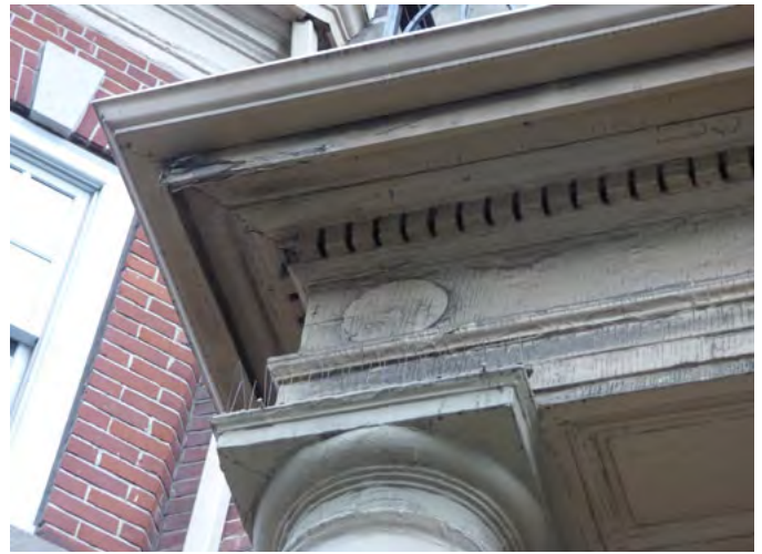
18. Condition of fascia and top of column at entrance portico. (ERA, December 2025)
