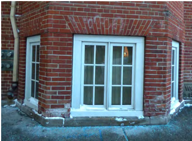
5. Efflorescence observed at base of projecting bay with snow build-up present (ERA, January 2026)
