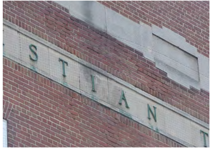
2. Areas of eroded joints and stained artificial stone at 4th floor and parapet wall (ERA, December 2025)
