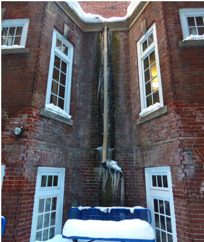
49. Failed downspout with surrounding organic growth and efflorescence at interior court space at grade (ERA, January 2026)
