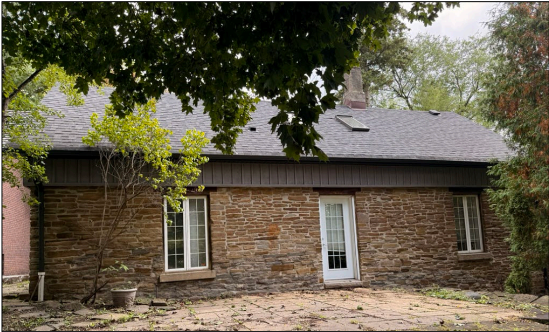
Figure 12: 34 Jason Road, west facade, showing three openings with modified opening at centre for access to stone patio (Alex Corey, September 2025).
