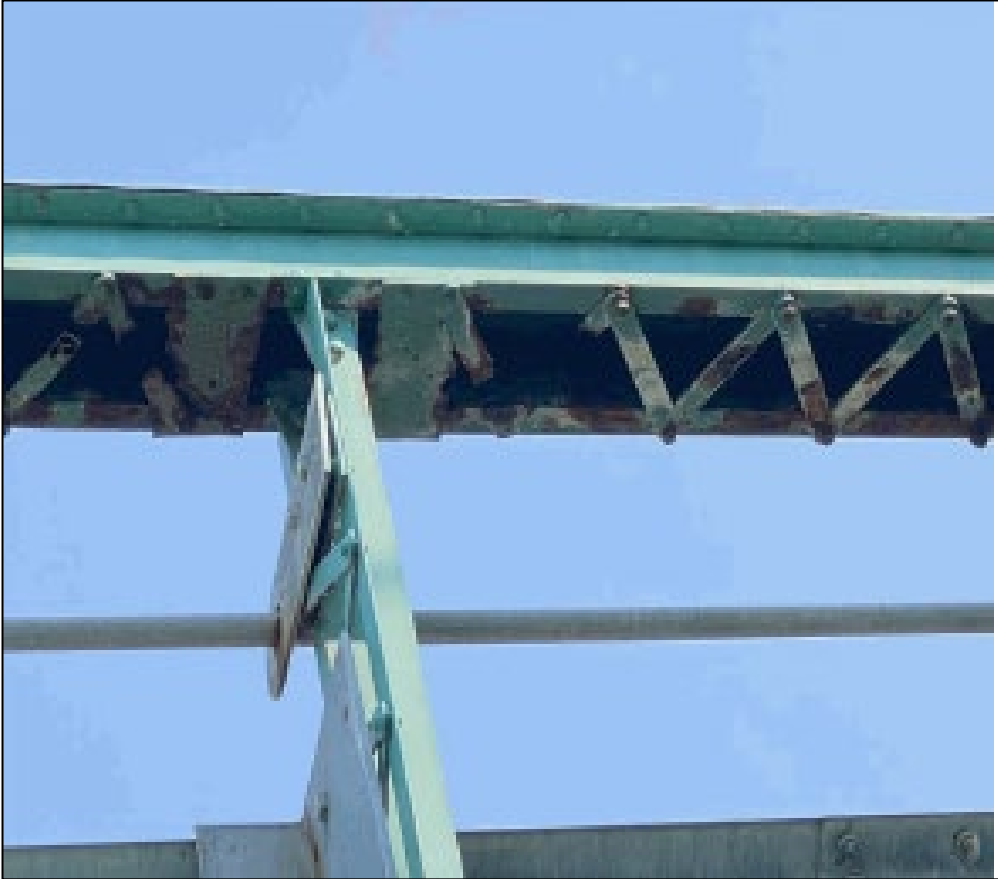
Detailed view of perforation in the tie bars on the top chord
