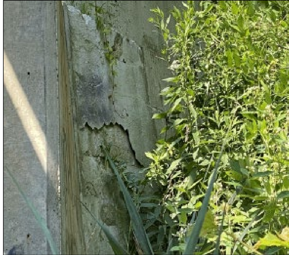
Detailed view of wide cracks and delamination on the wingwall
