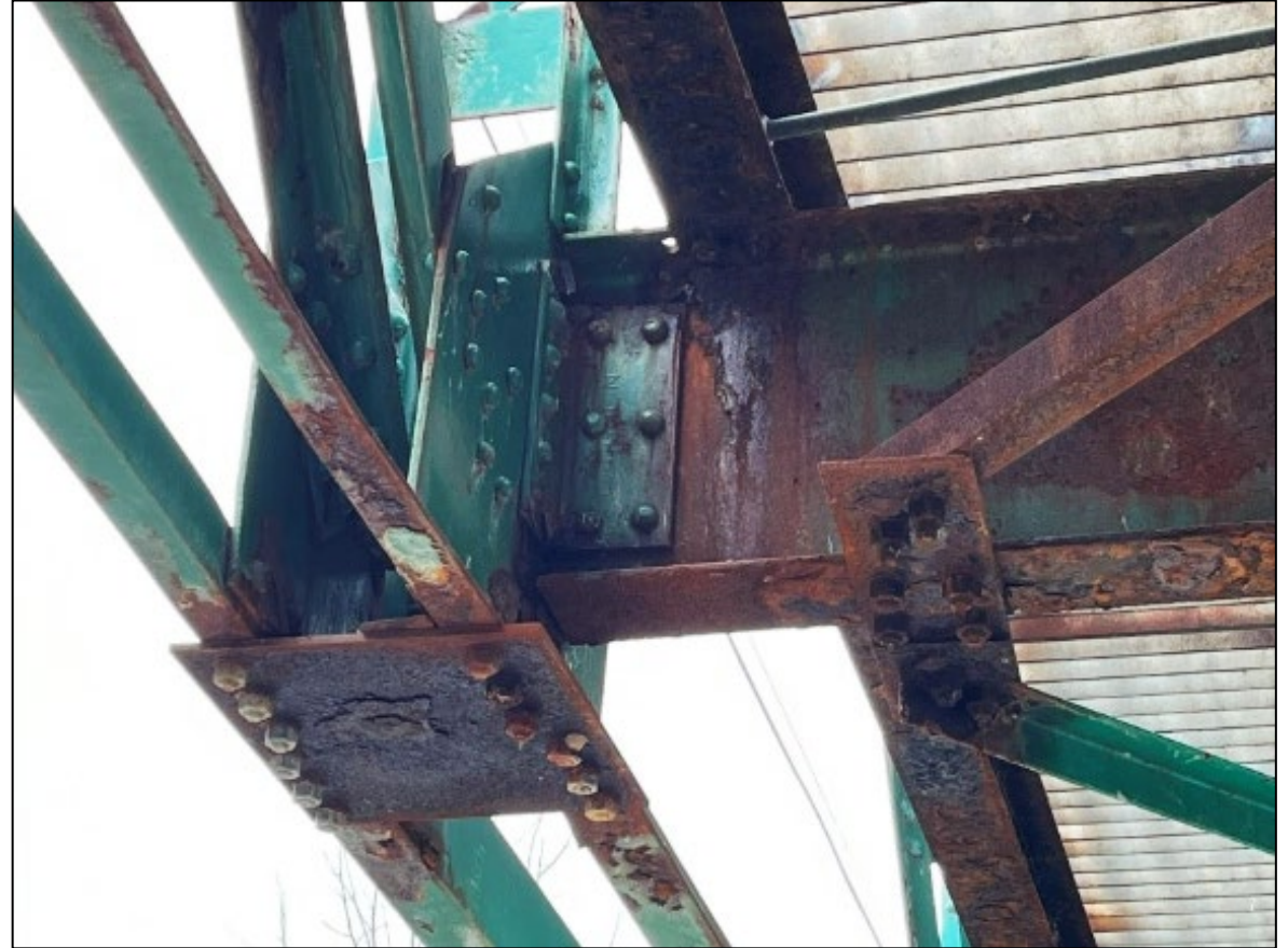
Detailed view of corrosion and severe flaking on the truss connections
