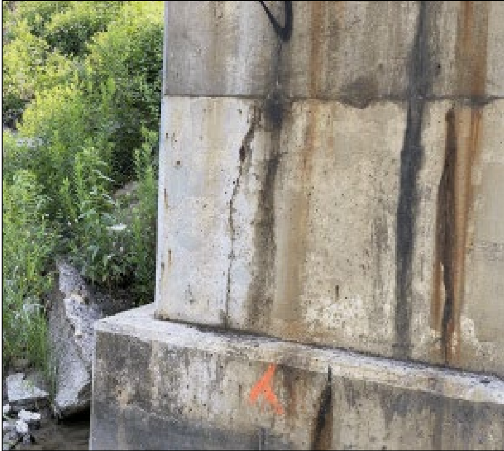
Detailed view of wide cracks and delamination on the abutment
