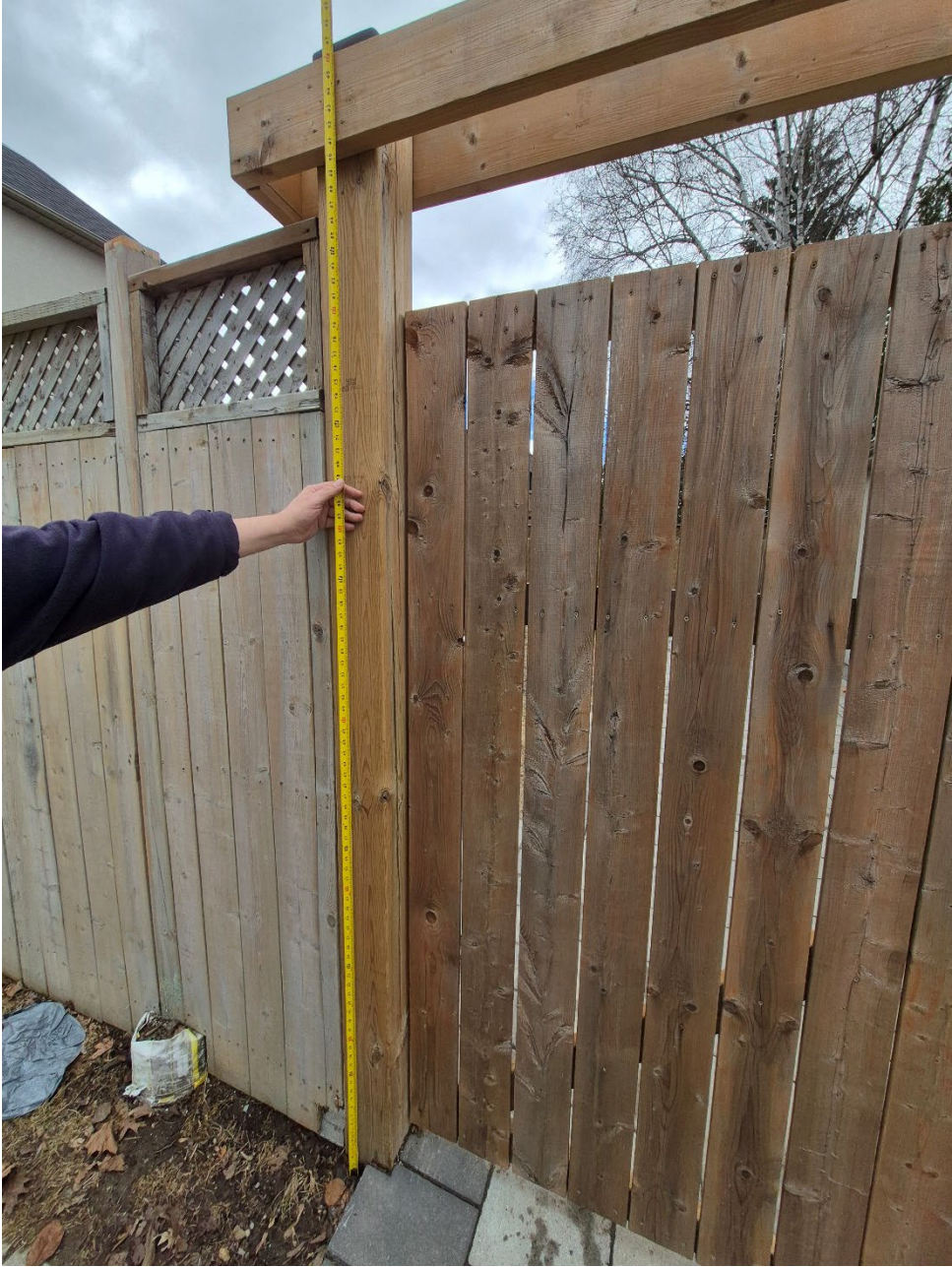
Attachment 3: Supervisor's photo - Fence Height (2.48 meters)
