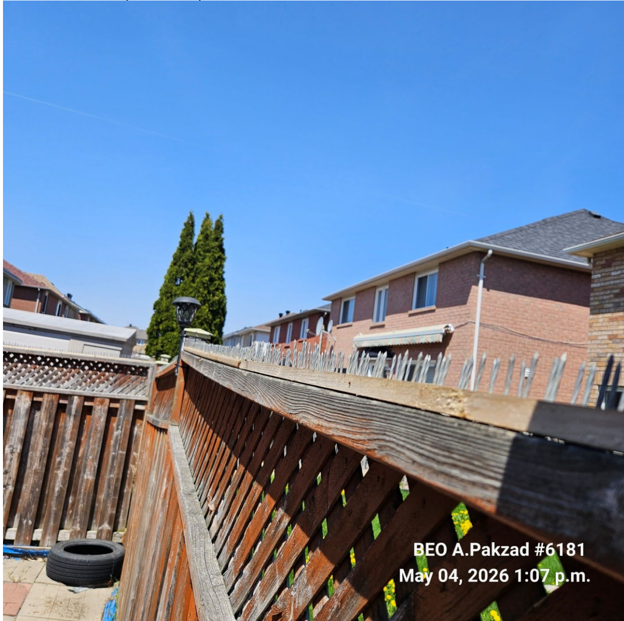
Attachment 5: Supervisor's photo – North side Fence Nails
