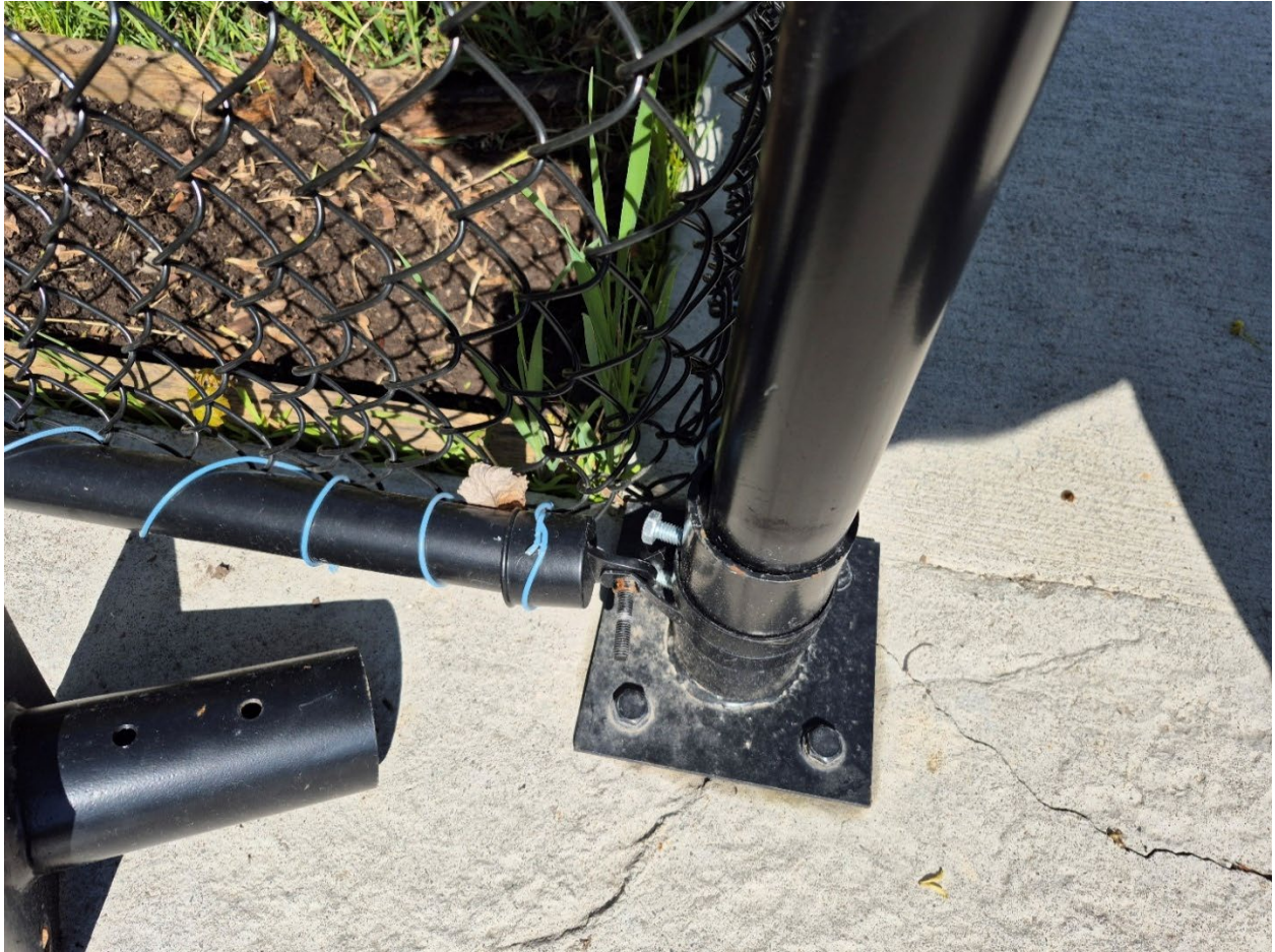
Attachment 5: Supervisor's photo – Pool Enclosure Fence Post (not embedded)
