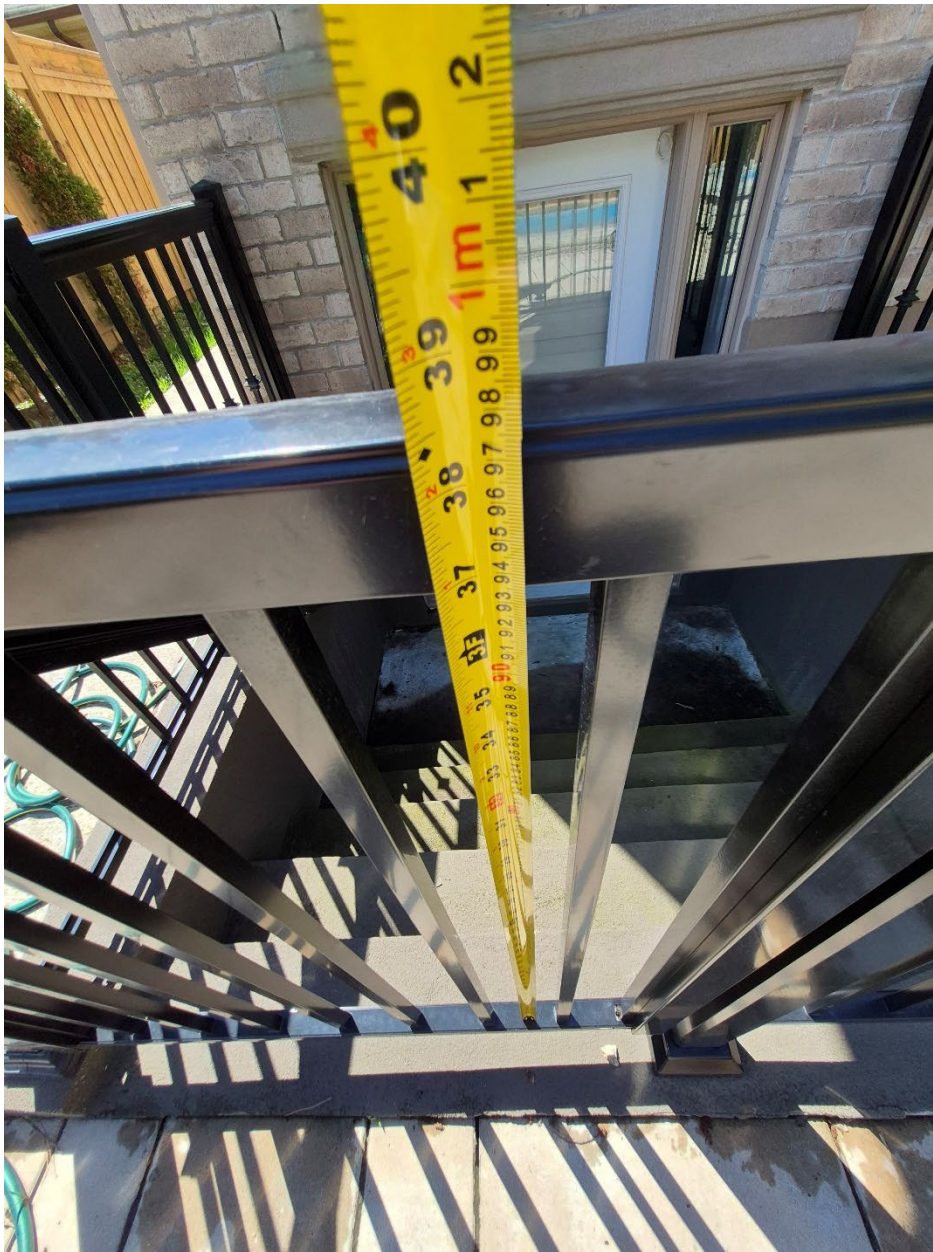
Attachment 11: Supervisor's photo - Fence in rear yard- northeast side of house - stairs to basement- fence height (0.94 meters)
