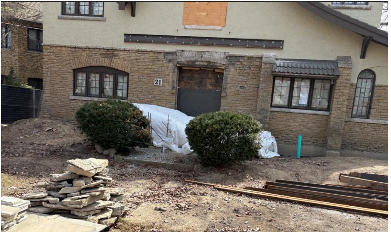
Photo of the front, north elevation of the existing building at 21 Baby Point Crescent after the removal of the preexisting door and entrance portico (City of Toronto, 2025).
