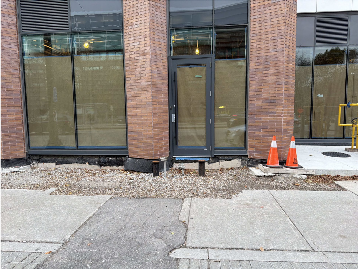
Attachment 5: Photo of Existing Condition facing the West Elevation of 666 Spadina Ave
