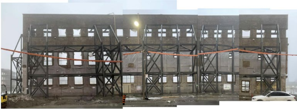
Figure 12: West elevation of the Warehouse Building, looking east (Giaino + Associates Architects Inc., 2026).
