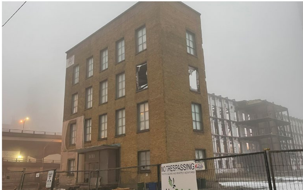
Figure 9: South and west elevation of the Office Building, looking northeast (Giaino + Associates Architects Inc., 2026).
