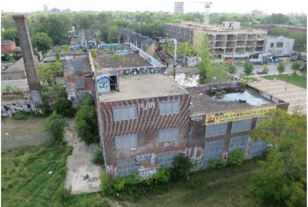
View of the north elevation, showing Building E and Building F (both not designated and proposed to be demolished) at 40 Wabash Avenue (SBA, 2024).
