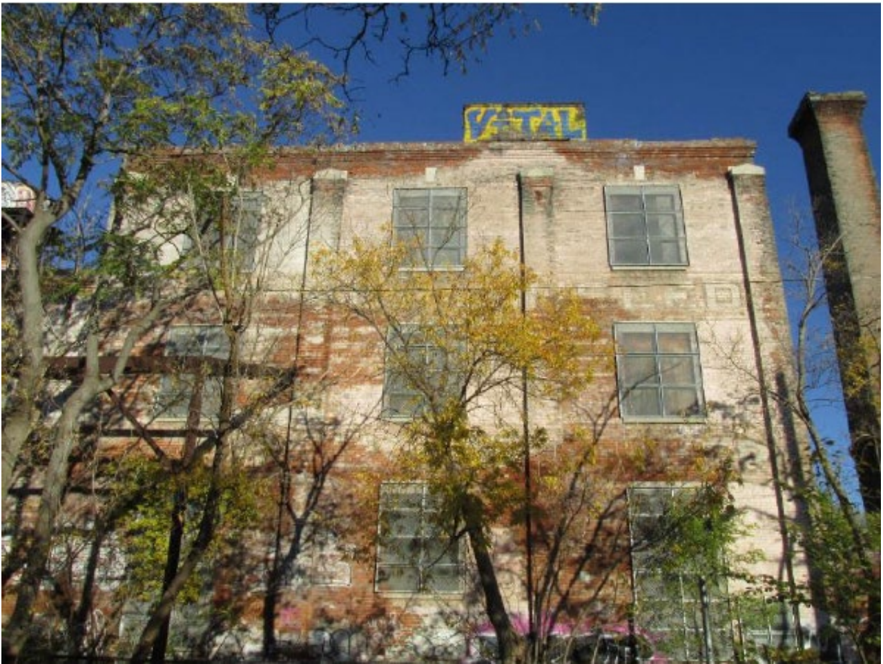
View of the south elevation, showing Building B at 40 Wabash Avenue (SBA, 2024).
