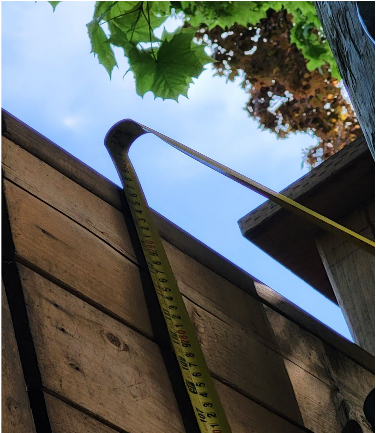
Attachment 10: Rear fence – West lot line – zoomed measurement confirmation from 292 Wright Avenue's grade
