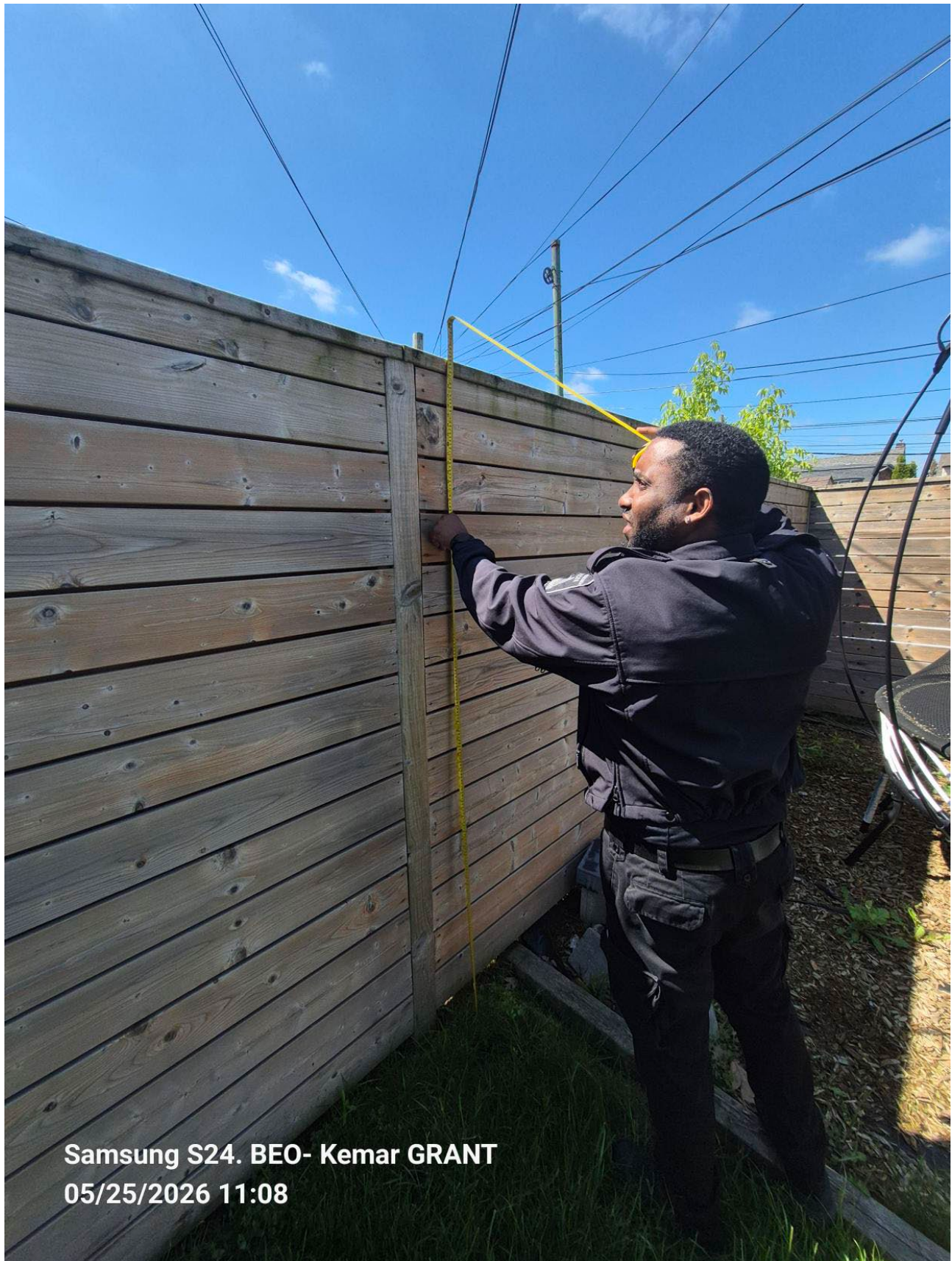
Attachment 9: Overview of rear yard- Eastern property line 3 rd and 4 th fence panel
