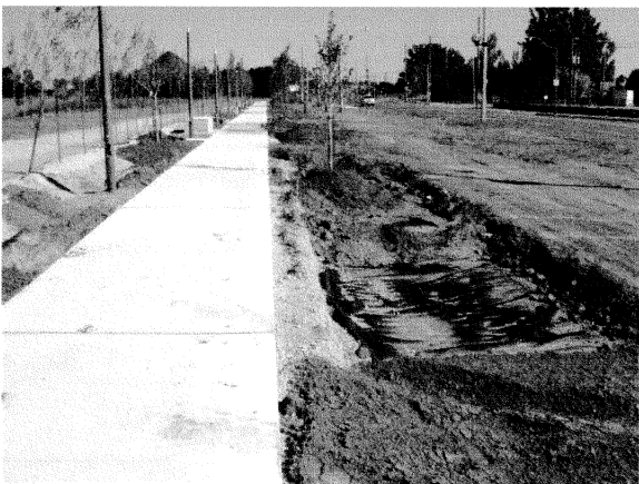
5- Geotextile in shallow excavations on the west side of the new sidewalk parallel to Leslie Street.
