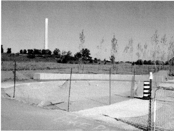
1 – View of new plaza area located on the southeast corner of Lakeshore and Leslie.
