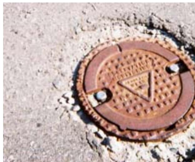
Monitoring well cap
