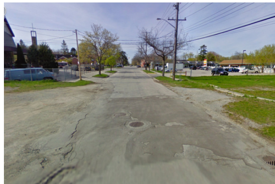
Streetscapes along the streets in the Village are in deteriorating conditions. Significant streetscape improvements are needed.
