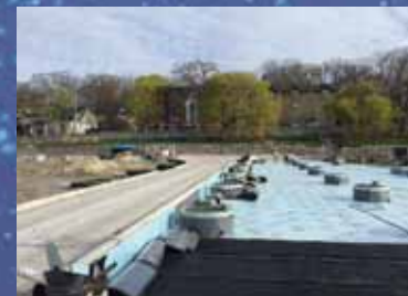
Existing Settling Basins Roof with Waterproofing (not visible), Insulation and (Black) Water Drainage Layer
