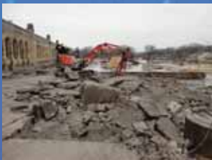
Demolishing of Road to Create a New Structurally Sound Road with Wider Curves for Delivery Trucks
