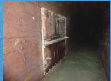
Temporary Closing of the gate Opening to Isolate the Basin for Rehabilitation Works
