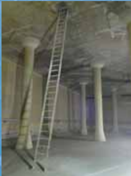
Old Access Ladders (6 m high)
