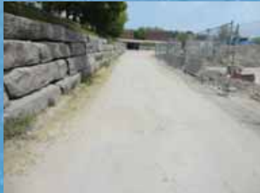
Existing Road to be Demolished and Re-Constructed, Including Better Drainage of Road and Basin Roof
