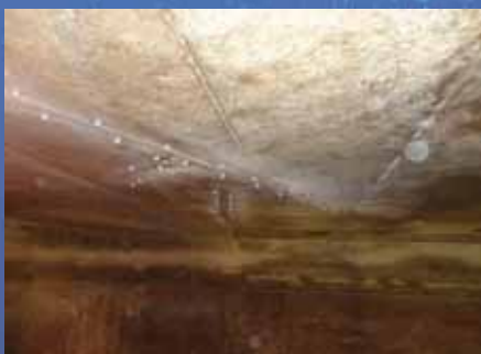
Cracks Inside the Settling Basin Concrete Ceiling. Crack Repair by Means of Injection with Caulking Material.
