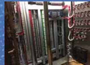
New Control Panel for the Automation of the Clean In Place System
