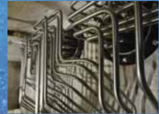
Hydraulic Piping to Control Clean In Place Valves Remotely
