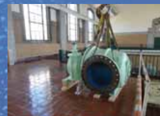
Refurbished Cone Valve
