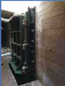
Newly Installed Basin Outlet Gate
