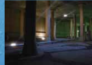
Newly Installed Stainless Steel Clean In Place Piping in one of the Settling Basins
