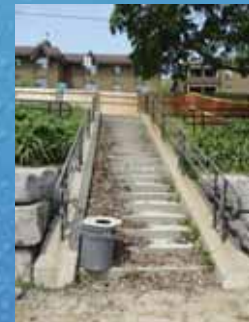
Old Concrete Stairway to be Re-Constructed to Current Standards
