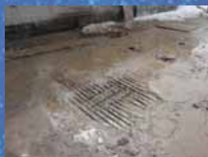
Damaged Existing Roof Slab, Exposing Rebar Underneath the Old Elevated Concrete Ring Road
