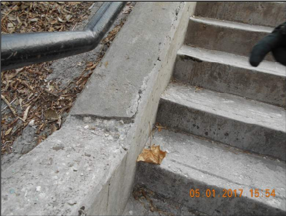
Photo 18: Spalling of Patch on North Stair Curb
