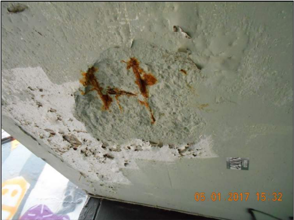
Photo 15: Spall at North Entrance Soffit
