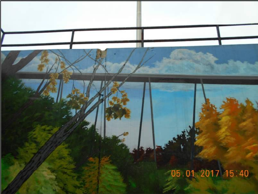
Photo 17: Crack and Spall in South Retaining Wall
