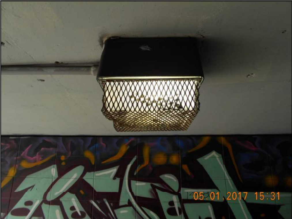
Photo 6: Typical Light Fixture
