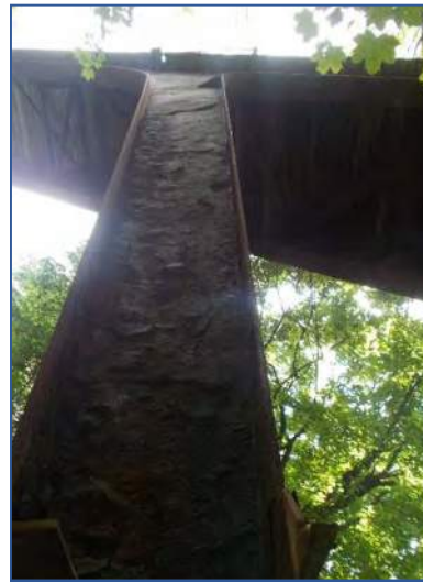
View of corrosion on inclined leg
