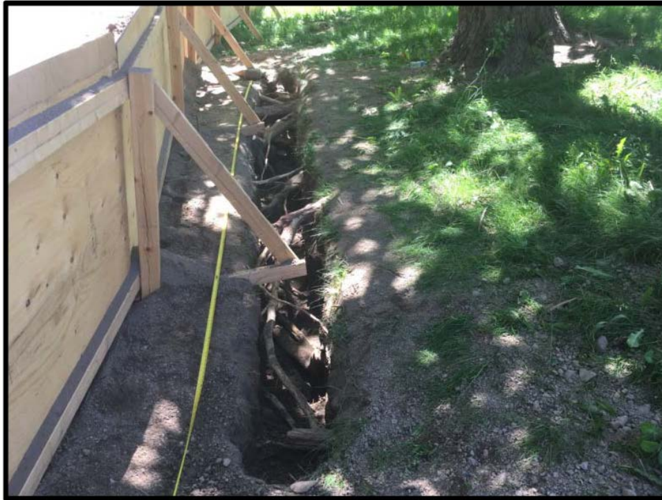
Tree Root Exploration Trench: After surface excavation, a vacuum removes soil to expose tree roots.
