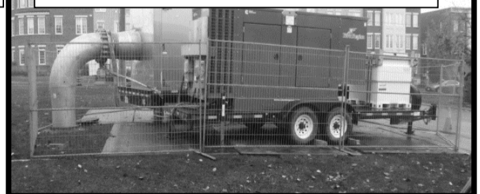
Photo 2 – Portable odour control unit
