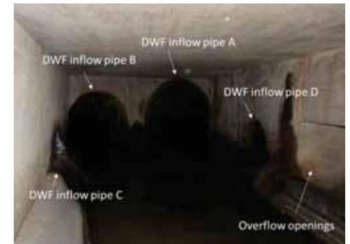
Overflow structures divert, or bypass flows to relieve an overloaded sewer (Shown: Hillary Combined Trunk Sewer Overflow Structure)
