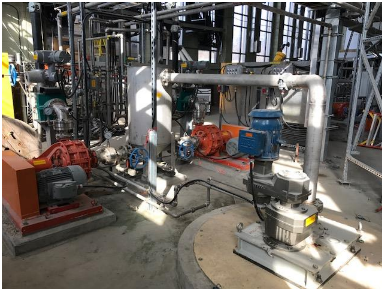
Figure 6 Vortex Grit Removal Equipment
