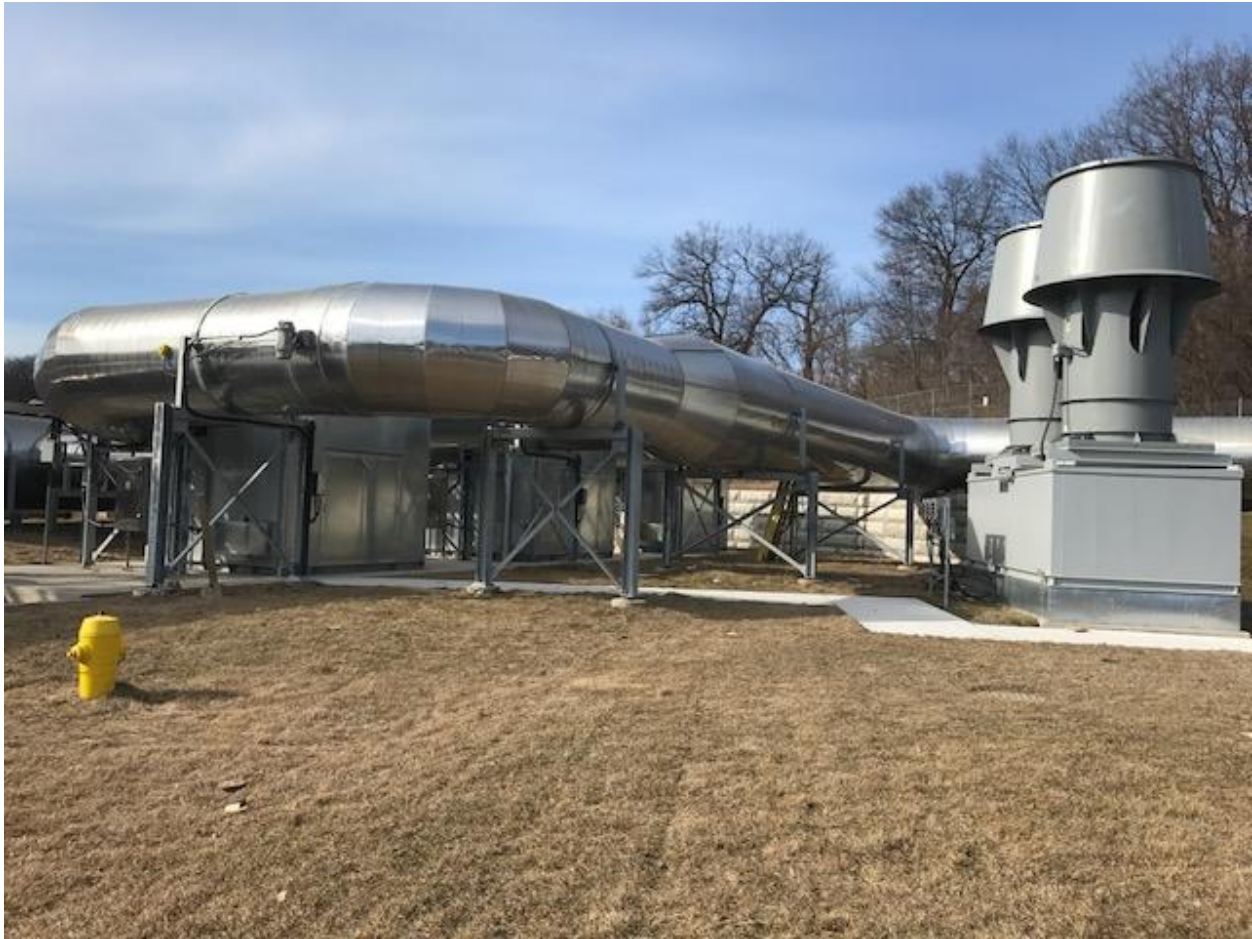
Figure 1: The Central Biofilter
