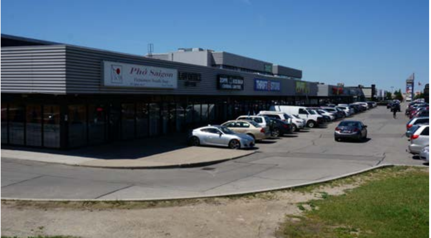
Strip mall condition (Merchant's Flea Market building) at Eglinton Avenue East and Warden Avenue
