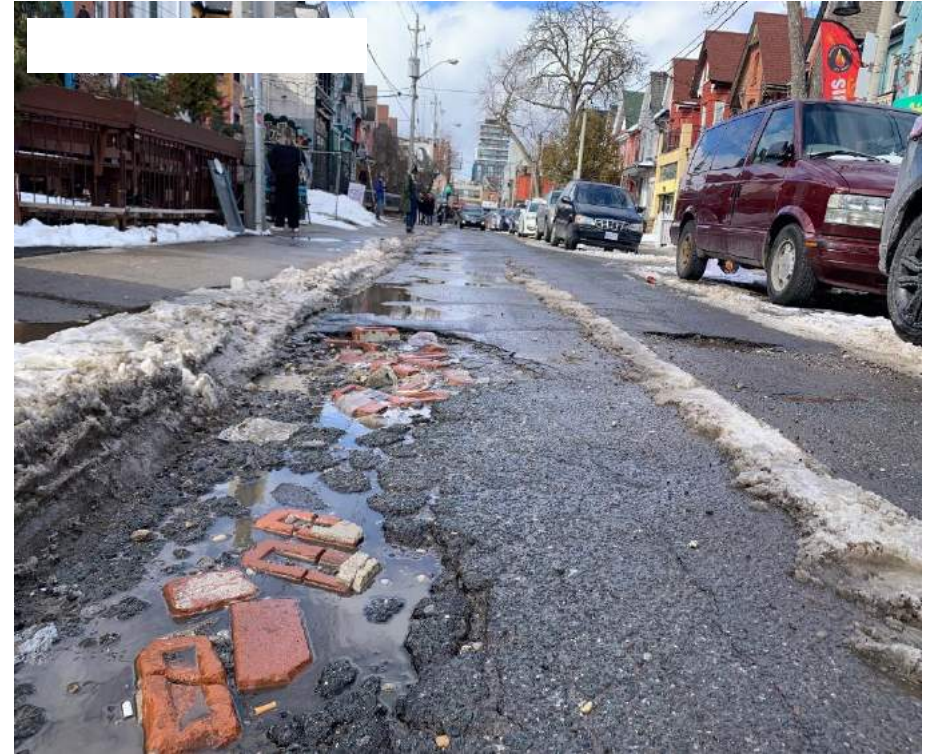
Kensington Market's roadway, curbs and sidewalks are aging and in need of major repairs.
