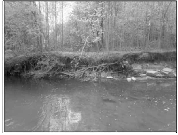
Erosion around a sanitary sewer
