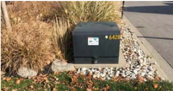
Padmount Transformer or Switchgear
