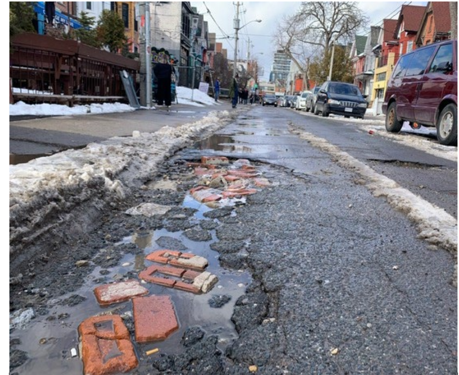
Poor condition of roadway on Kensington Ave
