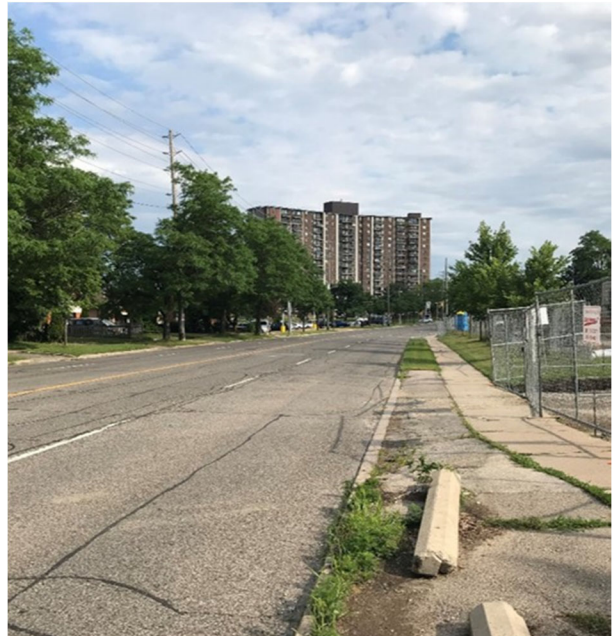
Figure 2: In Section A, there are two motor vehicle lanes per direction with minimum-width sidewalks. An asphalt boulevard in front of a school is in poor condition.
