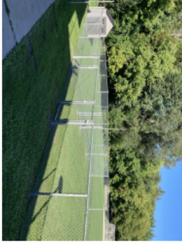
Example of Installation @ Bake Street Early Learning And Child Care Centre
