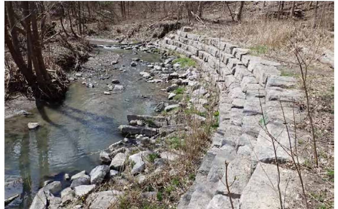
Photo of armourstone bank and vegetated stone treatment at the water's edge along the north stream bank of Burke Brook.
