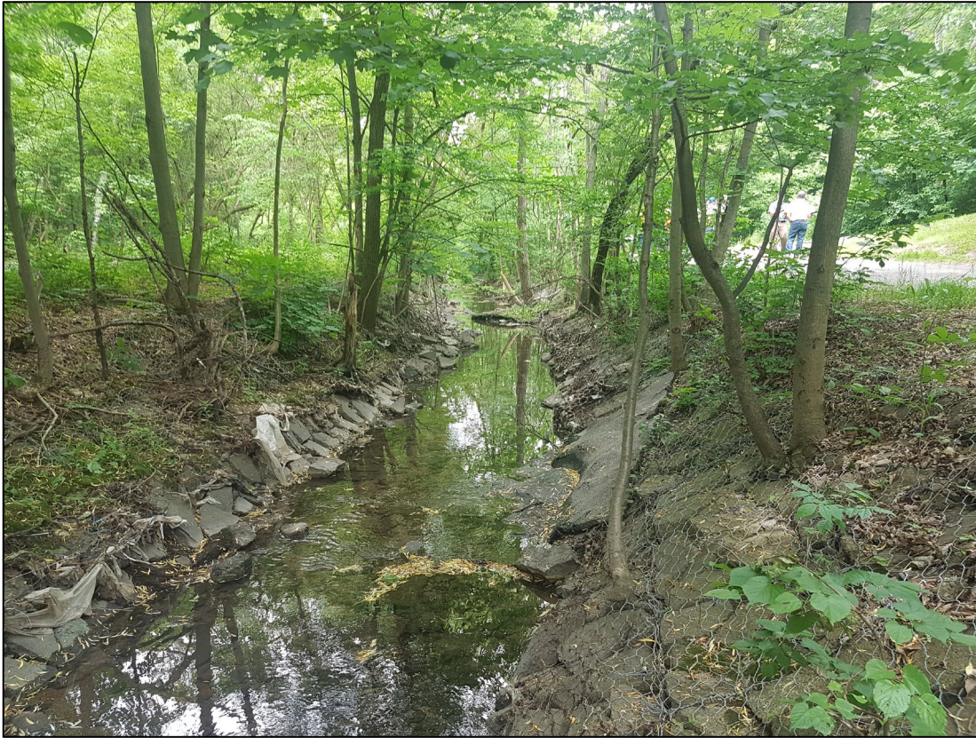
Duncan Creek Phase 2 – Deteriorated gabion lined channel (pre-construction)
