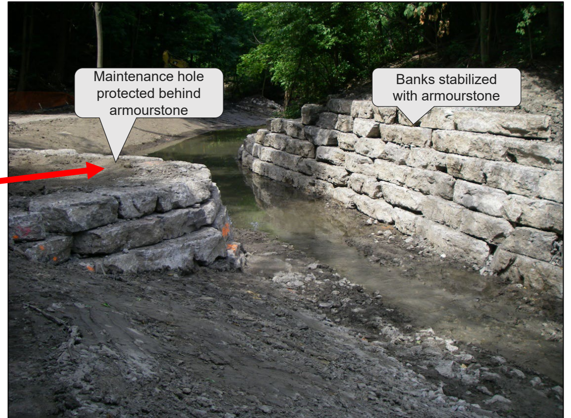
Massey Creek – Creek has been realigned away from maintenance hole with Armourstone walls built as bank protection (post-construction but pre-restoration)
