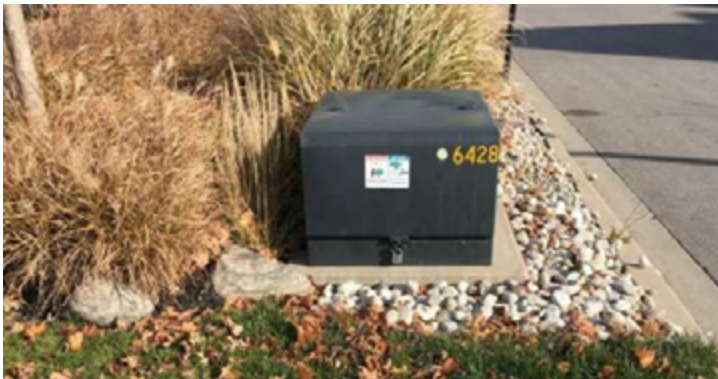
Padmount Transformer or Switchgear
