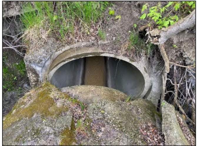
Photo 4: Site 58-41, failed outfall and eroding banks
