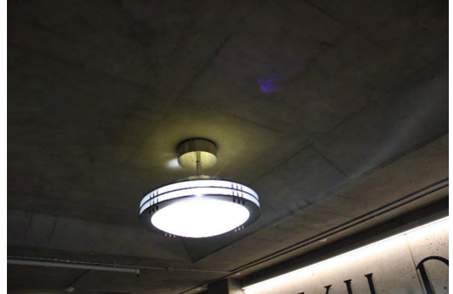
Plate 30: View of a light fixture illustrating the Art Deco influences within the north concourse area.
