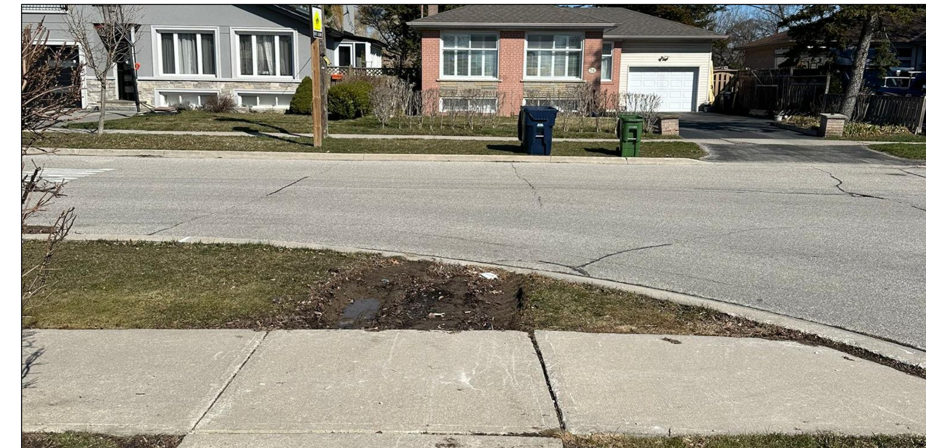
Missing sidewalk connection
