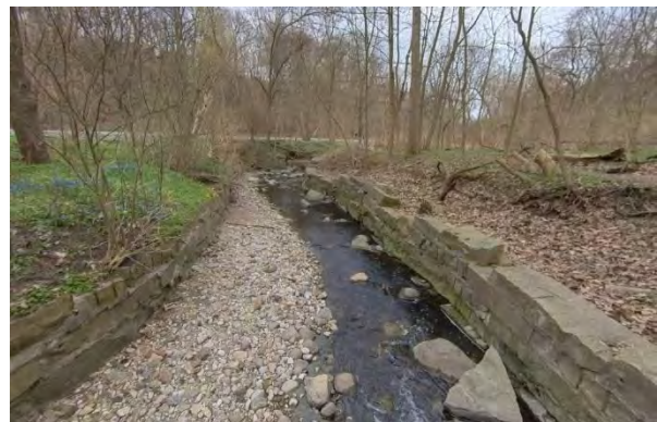
Photo 4.2 Facing east. Armourstone lined banks with erosion behind wall on right bank.
