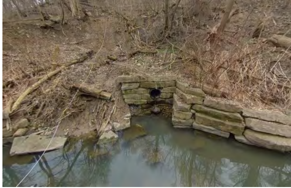
Photo 2.3 Facing west. Stormwater outfall on right bank with failing headwall and surrounding armourstone walls. Slope failure behind outfall. Large downstream erosion scars on the right bank.
