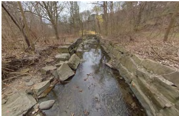
Photo 3.5 Facing south. Armourstone lined banks with failure on left bank.
