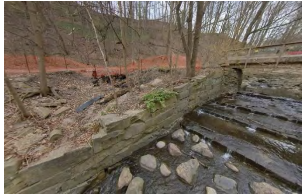
Photo 3.2 Facing west. Erosion and exposed geowebbing on right overbank.
