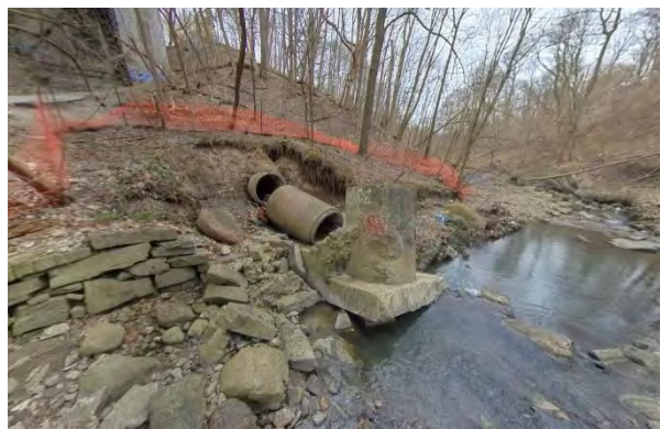
Photo 2.1 Facing south. Failed stormwater outfall on left bank.
