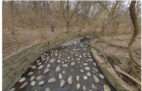
Photo 2.12 Facing east. Concrete bed embedded with roundstone. Evidence of scour behind armourstone wall on right bank.
