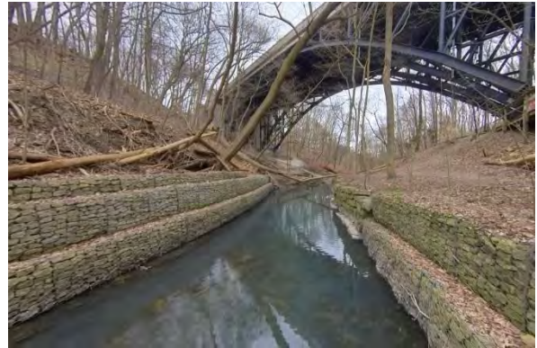
Photo 1.8 Facing south. Gabion baskets on both banks are stable but shows signs of degradation.
