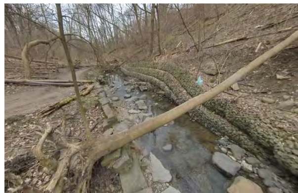
Photo 2.2 Facing south. Collapsed gabion on right bank and partially outflanked armourstone wall on left bank.
