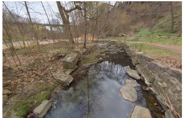
Photo 3.6 Facing south. Armourstone lined banks with failure on left bank.
