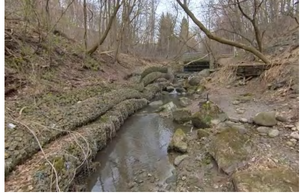
Photo 1.2 Facing north. Outlet of Yellow Creek at the upstream limit of the aboveground portion of the creek. Gabion baskets failing along both banks.
