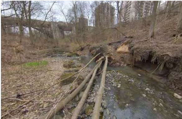
Photo 1.5 Facing south. Historical armourstone channel visible in left side of photo. Creek migrating west into valley wall resulting in severe scour and loss of mature trees.
