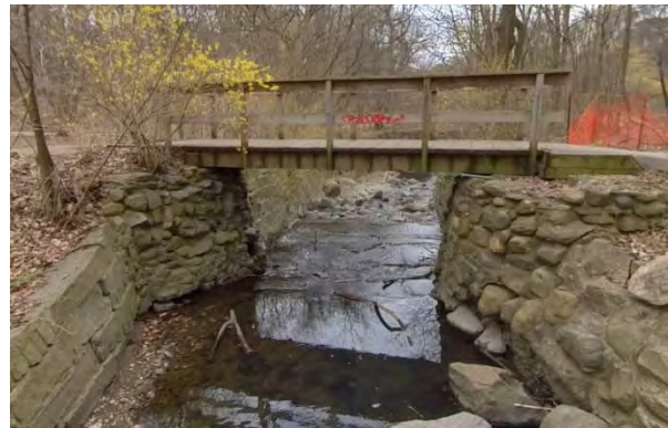
Photo 2.14 Facing south. Wooden pedestrian crossing. Abutments on both banks are undermined.
