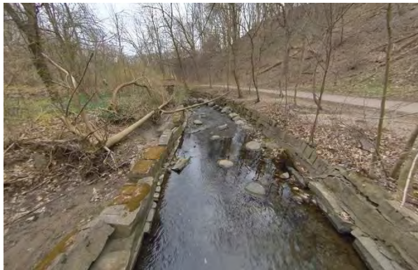
Photo 2.13 Facing south. Armourstone lined banks with evidence of scour behind wall on left bank.
