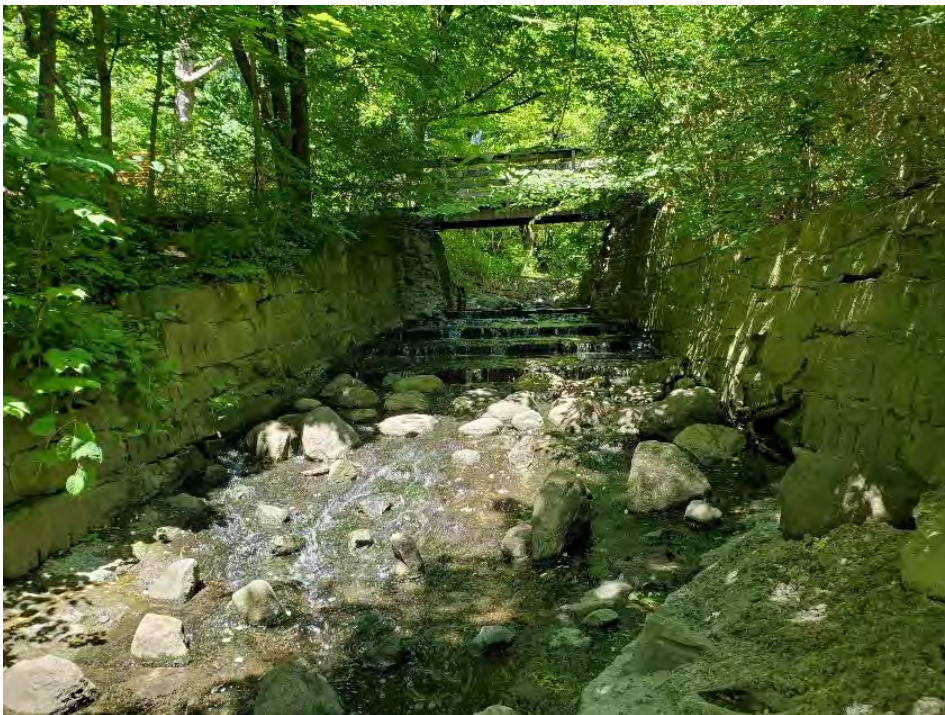
Pedestrian bridge, grouted quarried stone walls and instream boulder treatments observed in 2020
