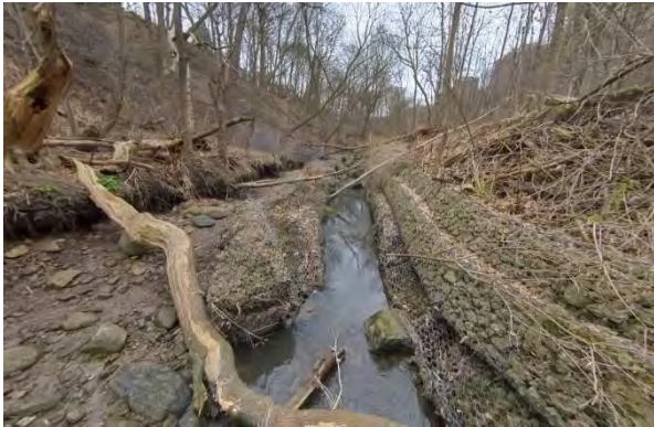
Photo 1.3 Facing south. Undermined and outflanked gabion baskets failing along both banks.
