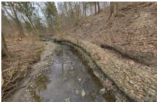
Photo 2.7 Facing south. Undermined and slumping gabion baskets on right bank.
