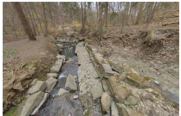
Photo 2.8 Facing south. Outflanked armourstone wall and failed concrete bed.
