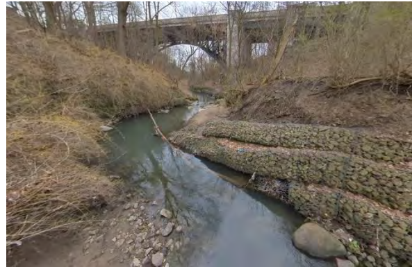
Photo 1.6 Facing south. Collapsed gabion on right bank due to undermining and scour behind the wall.
