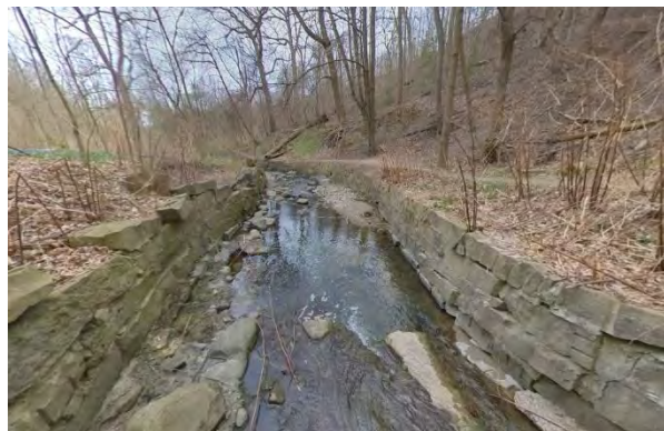
Photo 4.1 Facing south. Armourstone lined banks with displaced armourstones on left bank.
