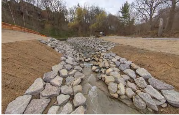
Photo 3.7 Facing north. Headcut/knickpoint migrating upstream through the exposed till.
