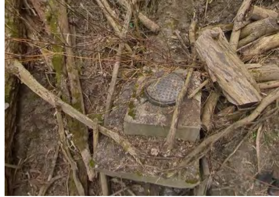
Photo 2.4 Facing west. Storm sewer pipe connecting to maintenance hole is exposed due to loss of material associated with slope failure.
