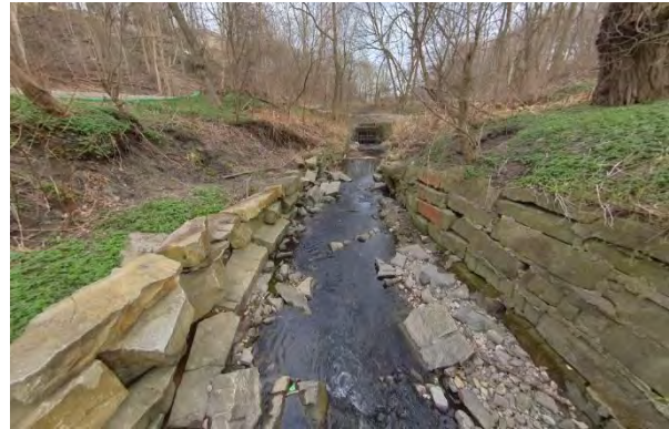
Photo 4.6 Facing south. Armourstone lined banks with failure on left bank.
