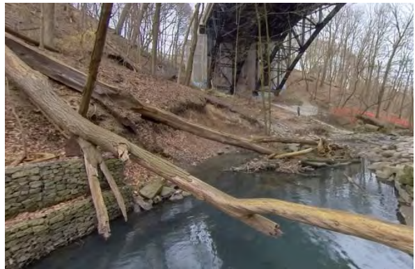
Photo 1.9 Facing south. Large erosion scar on left bank downstream of gabion.
