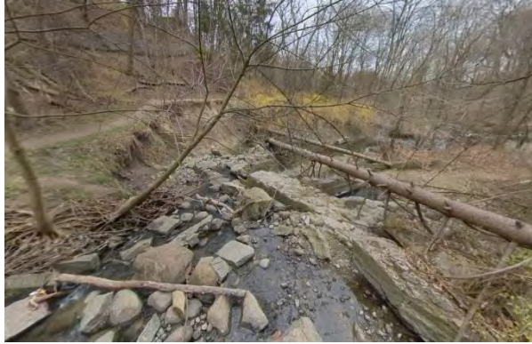
Photo 2.9 Facing east. Outflanked concrete spillway in the foreground and large erosion scour in the background.
