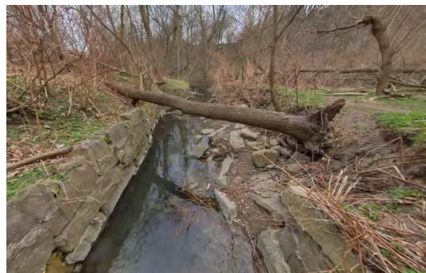
Photo 4.4 Facing south. Armourstone lined banks with failure on right bank.
