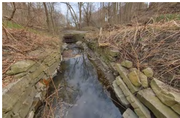
Photo 4.7 Facing south. Armourstone lined banks with failure on right bank.
