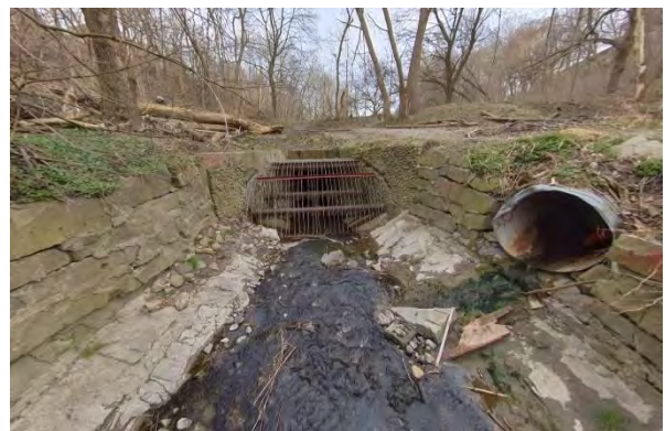
Photo 4.8 Facing south. Downstream inlet structure. CSP culvert conveying overland flow on right bank.
