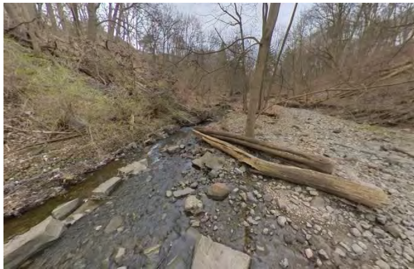
Photo 2.5 Facing south. Flood flow channel and cobble bar visible in right side of photo. Creek migrating east into valley wall resulting in collapse of gabion on east bank.
