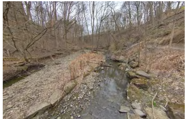
Photo 2.6 Facing north. Flood flow channel and cobble bar visible in left side of photo. Creek migrating east into valley wall resulting in collapse of gabion on east bank.
