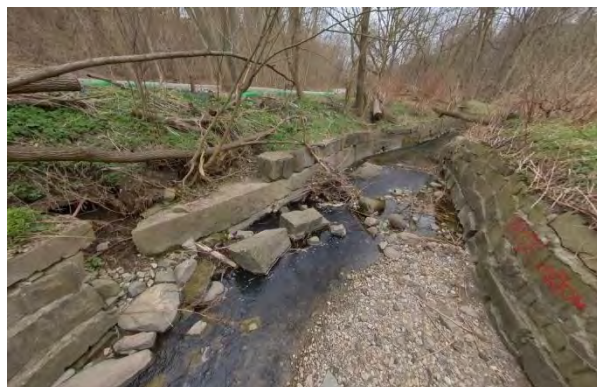
Photo 4.3 Facing south. Armourstone lined banks with failure on left bank.
