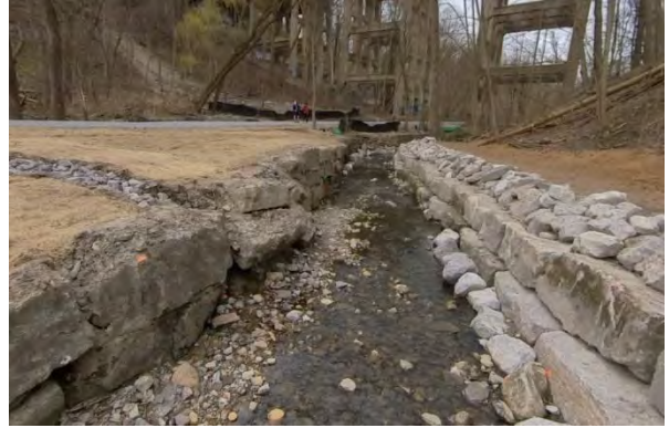
Photo 3.8 Facing south. Failing armourstone wall on left bank.
