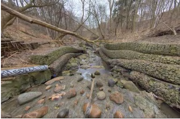
Photo 1.1 Source outfall, facing south. Failed concrete apron and failed gabion bank treatments. CSP outlet on left bank.
