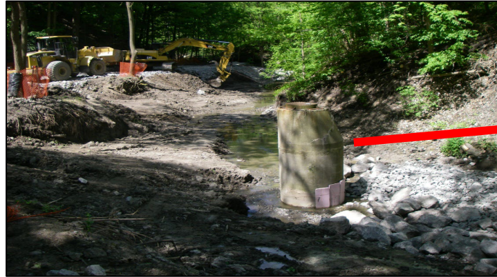
Taylor-Massey Creek exposed maintenance hole (during construction)
