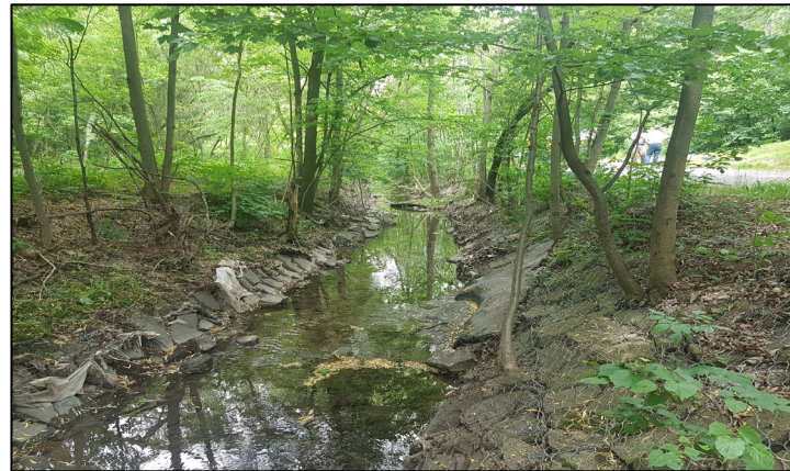
Duncan Creek – erosion accelerated by large storms and exposure of water infrastructure
