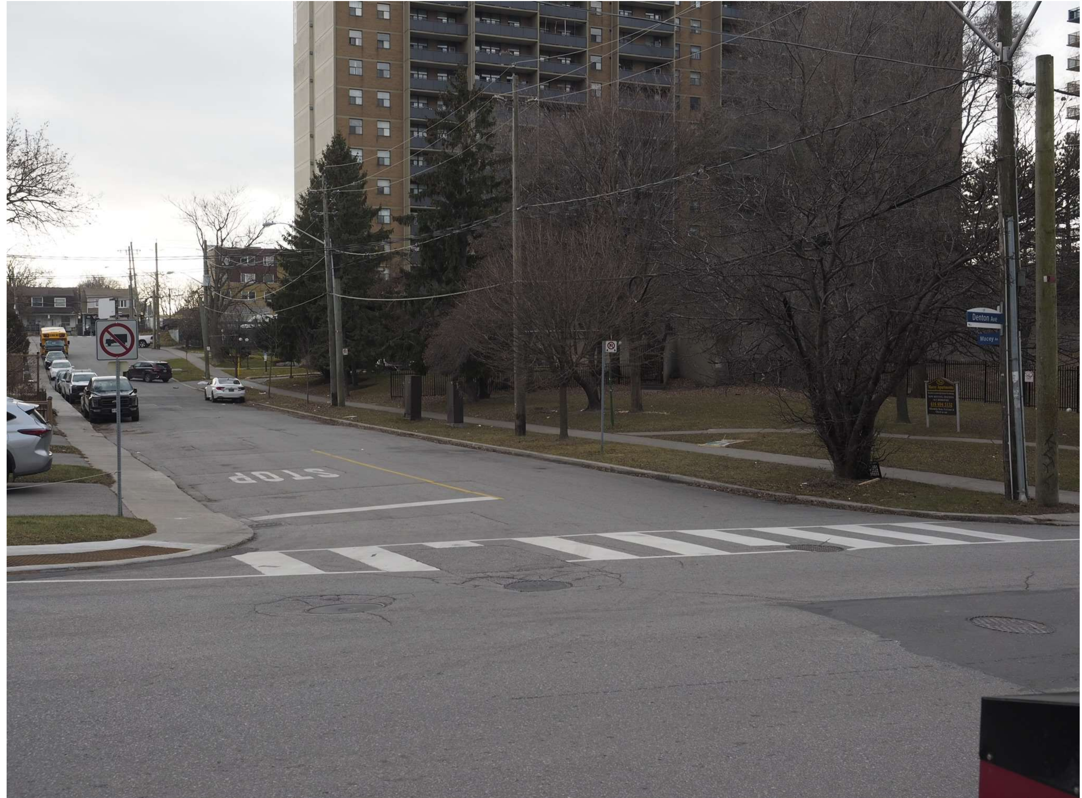
Faded pavement marking at Denton Avenue and Macey Avenue
