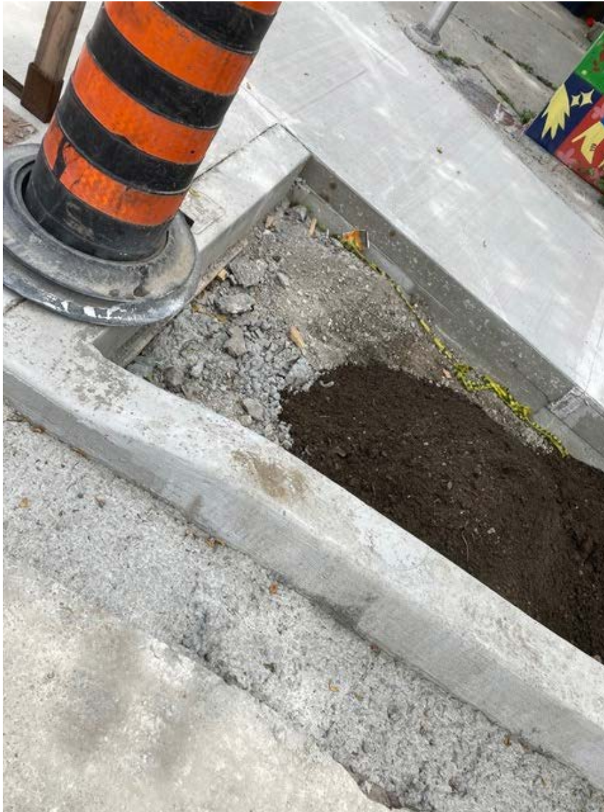
Figure 15: Cement / concrete debris and sediment contamination of bioretention bed will impact stormwater management function and health of the plants.
