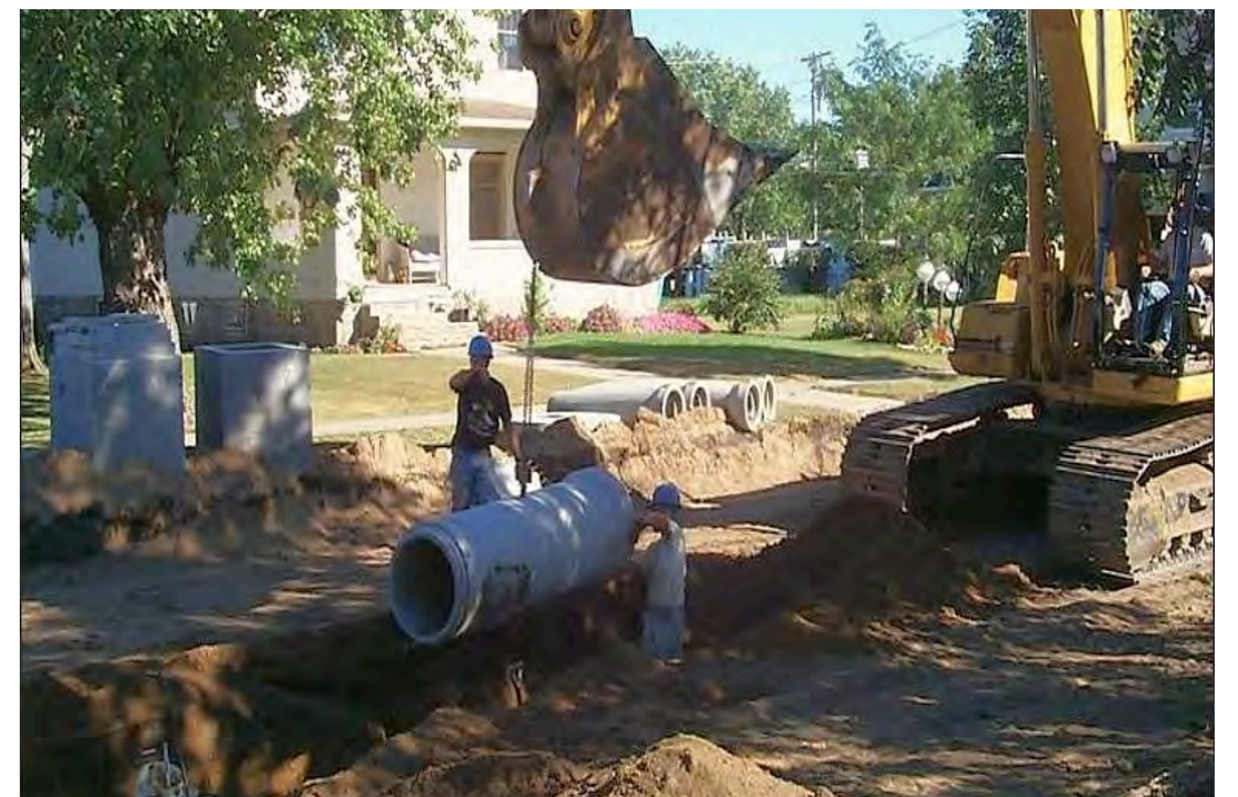
Sanitary and storm inline storage and storm sewer upgrades projects have already been constructed in the Growing Marlee-Glencairn Study Area.
