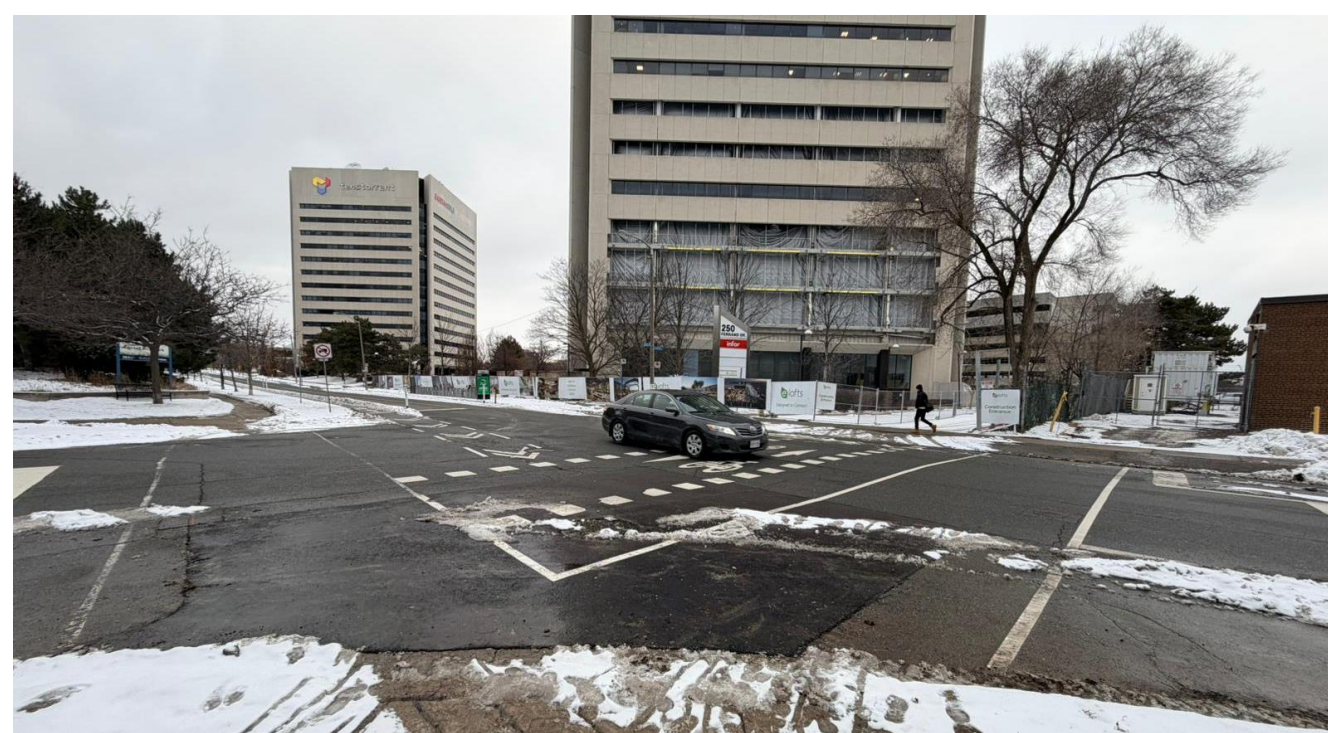
Missing zebra markings at the intersection of Deauville Lane and Rochefort Drive
