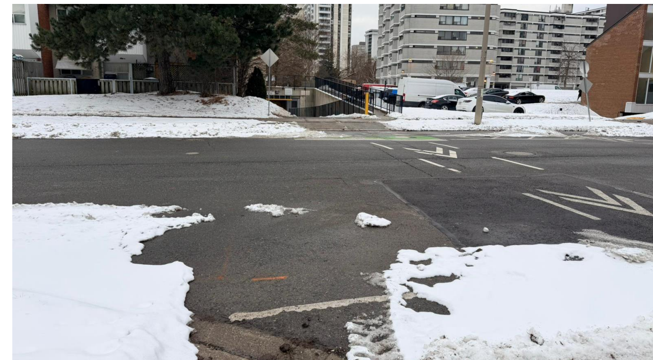
Missing crosswalk at the intersection of Rochefort Drive and Ferrand Drive
