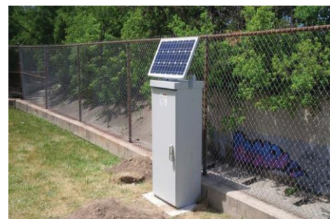
Real time water level gauge (located near Alliance Avenue)
